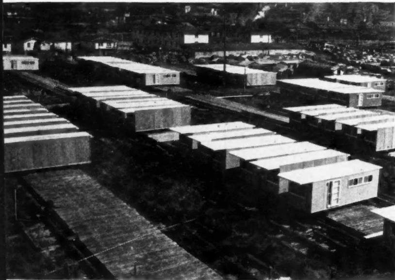
5 FINISHED SECTIONS go to storage yard. Here they await reloading on trailers for haulage as needed at the prepared foundations at building site or for shipment to a furniture factory for special built-in furniture to be installed.
