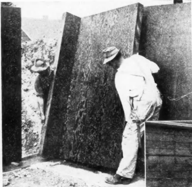
FIVE CENTS per square foot of wall for setting, stripping and cleaning compares with 35 to 40 cents the old way. Forms are re-used many times, producing perfect basement walls as shown at right. Details of construction above.
