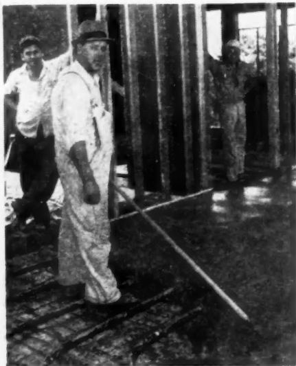
POURING slab on ground floor over gravel fill; 800 feet of 2" wrought iron pipe used for heating coils. Upper floor coils are 1 1/4" and slab rests on precast concrete joists; floors in all rooms finished with asphalt tile.
