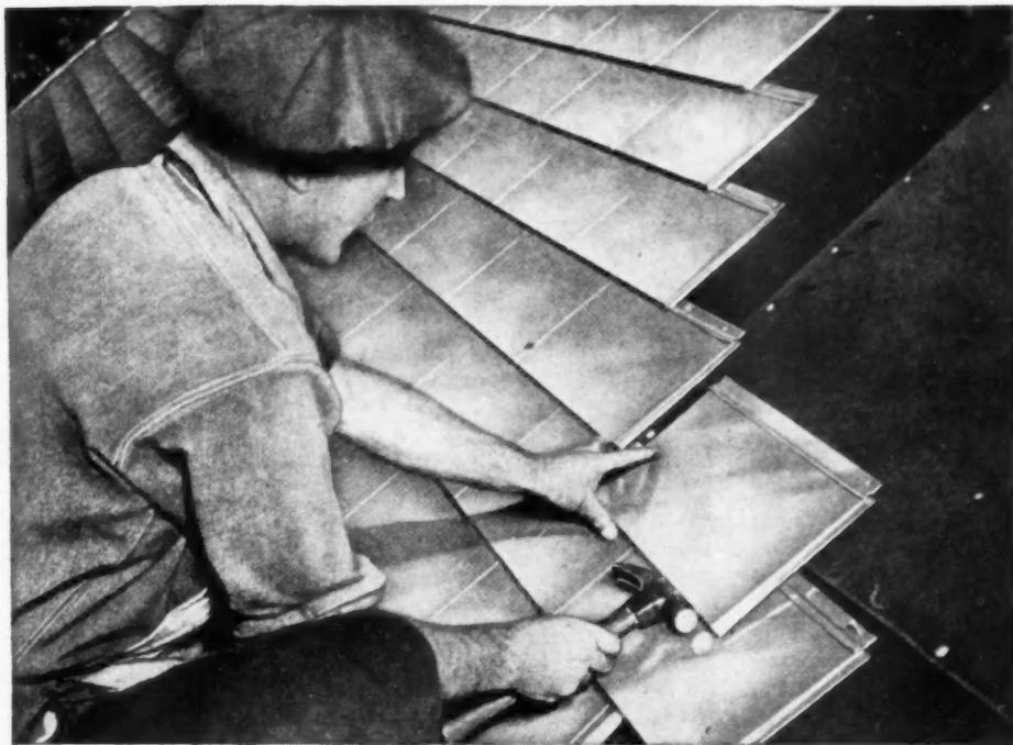
Reynolds Lifetime Aluminum Shingles being applied on a fine home in Kentucky. Note the attractive shadow line, the ease of application and simplicity of design . . . for a lifetime roof.
