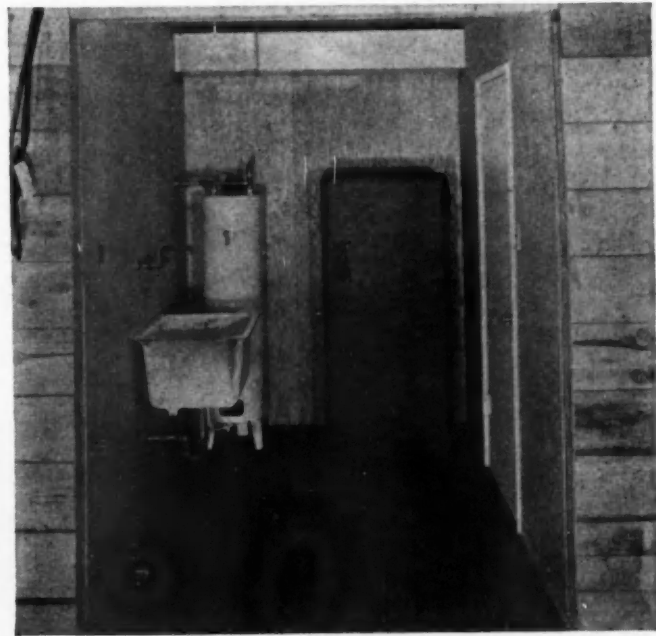
UTILITY room ready for use when Mobilcore is placed on foundation and service piping is connected. Utility core includes heating unit, laundry tray and domestic water heater.
