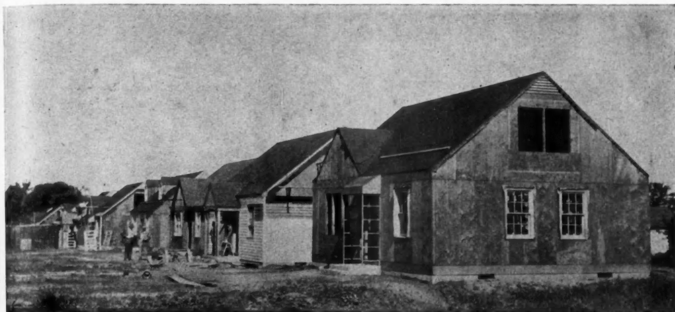
STREET scene showing Pomeroy houses in various stages of construction. Program calls for lathing and plastering in groups of ten.
