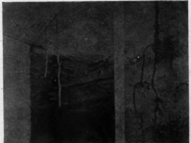
LEFT: Shelter tubes built down from above by termites in search of additional contacts with ground moisture. Right, termite tubes on a wall which did establish contact between a structure and ground moisture to permit termites to carry on their destruction.
