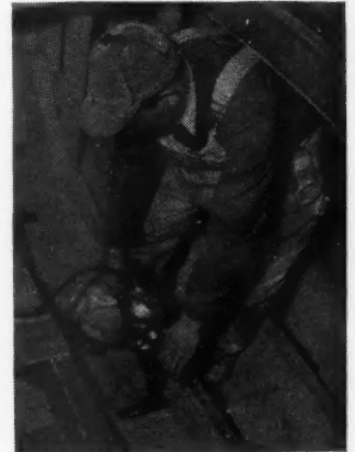
Electric drill with right angle drilling attachment for boring floor joists for pipe line. Photo: Black & Decker.
