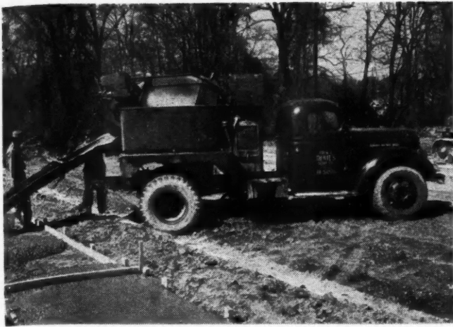
Mixing concrete in transit so it is ready for pouring on arrival at the building site is a big factor in time and labor saving. Photo: General Motors.
