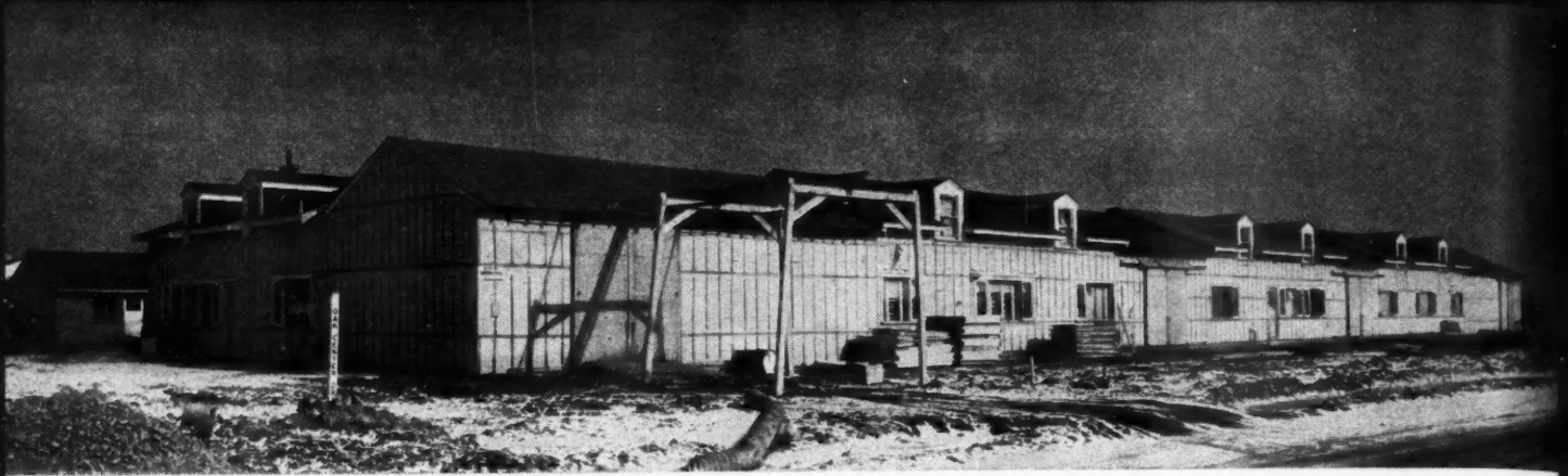
CONVENTIONAL houses are linked together with temporary enclosures to create a shop area to assemble panels and wall sections.
