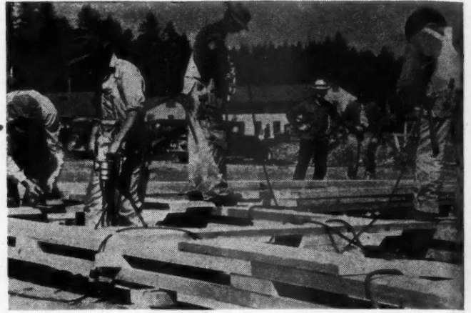
Today's high hourly wage costs call for maximum use of all types of portable power equipment on all types of construction jobs. Photo: Black & Decker.
