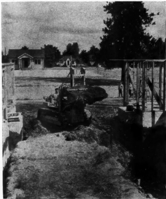
Small, crawler-type tractors with various dirt-moving attachments save today's home buyers many dollars and provide a more finished job. Photo: Caterpillar.
