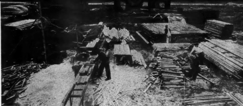
PRE-CUTTING of framing members on the site preparatory to use in assembly of wall sections.
