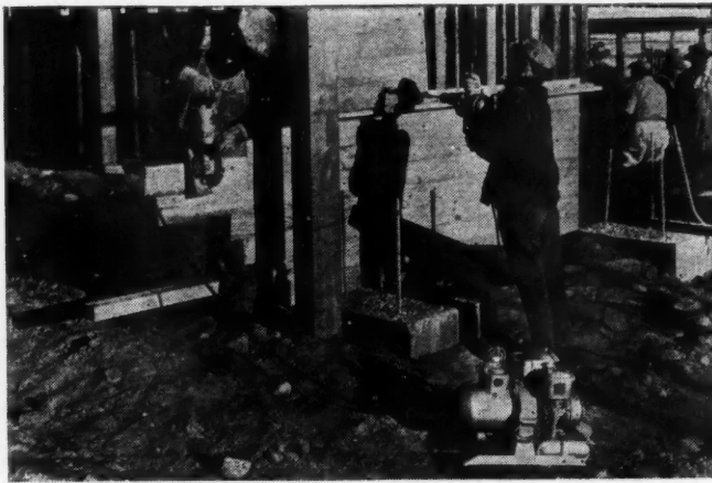
Where electrical lines have not been extended to job site, small portable electric generators are available to provide power for tools. Photo: Homelite.
