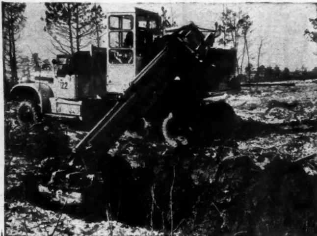
TRENCHING job shown above is one of the many performed by this multi-purpose earthmover, with its 24-foot telescoping boom.
