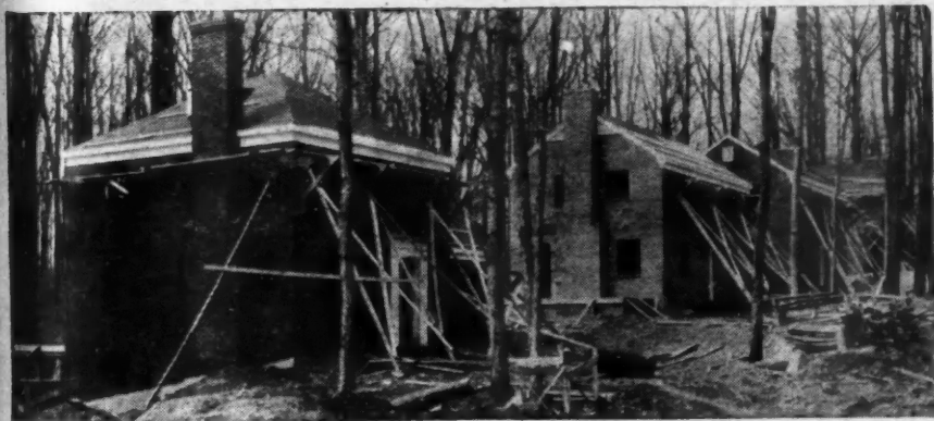
A VIEW showing construction under way on four of Glen Mar Park's 196 units.
