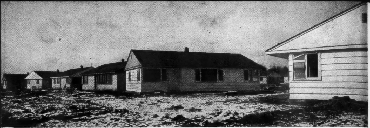
PARTIAL view of the development showing a group of the houses in various stages of completion. Street grading has not been done.
