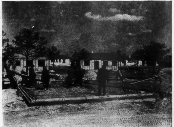
PHOTO shows concrete floor slab being poured over shop-fabricated and tested copper coils of the radiant heating system.
