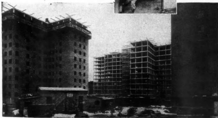
Truscon Diamond Metal Lath Used in Elliot Housing Project, New York City.
