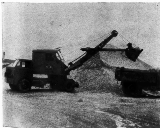
Handling of bulk aggregates and other materials with power equipment is a must with today's building methods and labor market. Photo: Harnischfeger.
