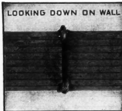
Enough mortar should be used to cause excess mortar to ooze out of the joints on both sides of the tile.
