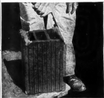
Method 1. Full head joints should be thrown onto both edges of the tile to be placed, or—
