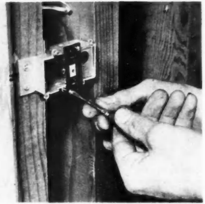
A workman installing a 25-volt switch. It is a single-pole, double-throw momentary control switch, normally left open
