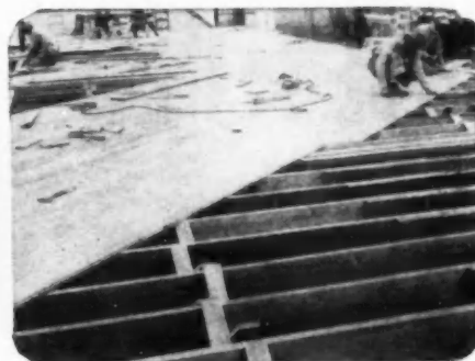
2. Wood used in or near the ground open to attack by termites.
