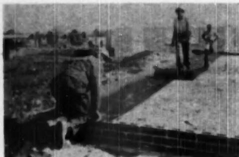
SPECIALIZED crews speed operations. Above: Applying 16-pound membrane waterproofing. Right: Slab is poured from mixer
