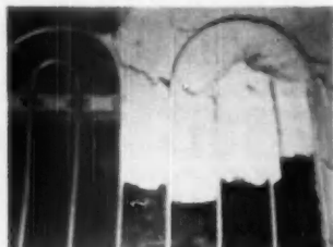
FIG. 4: Excess plaster and short strokes of trowel are necessary when coil is below the plaster base.
