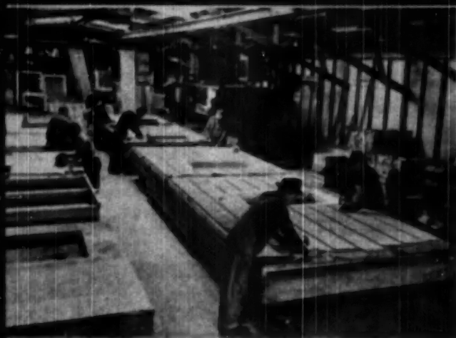
PRODUCTION carpenters finish five houses daily ready for assembly, in enclosed plant. Right, project developed with precut homes
