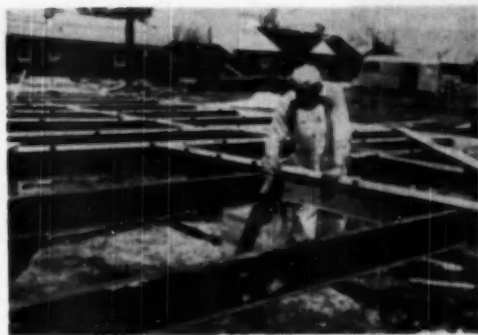
THE entire steel framework for the floor of this ranch-type home was assembled in less than half a day. Wood nailing strips on top of Junior Beams will hold two-inch subflooring and hardwood floors
