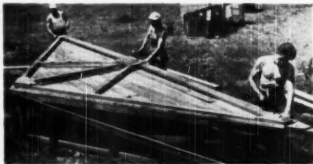
THIS is the simple truss, made up of 2x8's, 2x4's and plywood gusset plates, which was used in the 70 ranch houses in Green Acres. Trusses were assembled on a jig at the site
