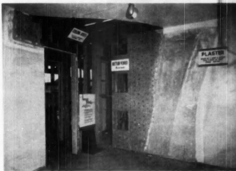
PROGRESSIVE steps in construction of wall are shown by labels attached to studs and underlappings of two coats of plaster and two coats of paint. Note heating unit.
