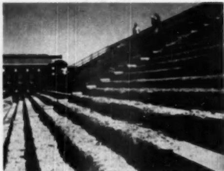
DETERIORATED tiers of Iowa State College Stadium were chipped and cleaned off to expose solid concrete for shooting new surface
