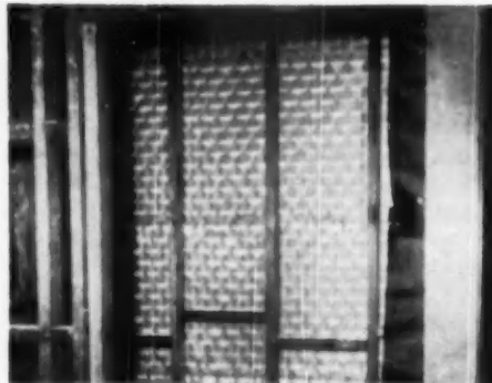
SPRAYED on with proper pressure, the plaster forms a strong key behind openings in the K-Lath, as illustrated here
