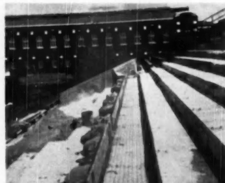
AFTER cleaning tiers of stadium, reinforcing mesh was formed on templates and put in place. Baffle boards to restrain spray were held in place with sand bags
