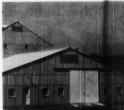
PARTICULARLY for larger buildings such as this barn, corrugated sheets are an excellent roofing. Specially formed units are used to protect the hips and ridges.
