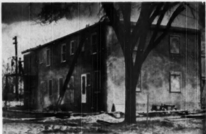
CONCRETE , reinforced with steel mesh, was shot against Masonite sheathing to form
