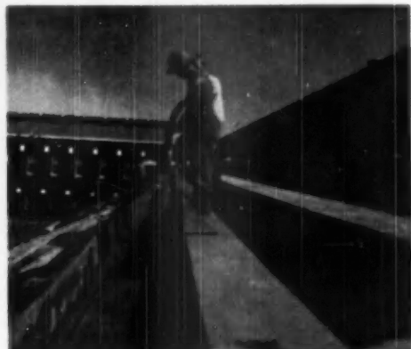
ONE COAT of pneumatically applied concrete was shot into place. ¾ to 1-inch thick. Layer and bond are stronger than original
