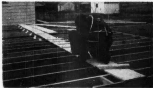
BRIDGING at the underside of joists is never nailed until the subfloor is nailed in place
