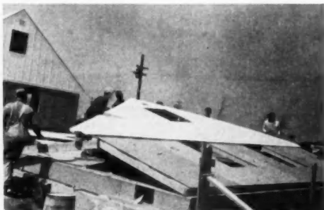
Men start raising gable end. Both ends are raised, braced and nailed in less than five minutes
