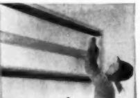
2. Check casing for plumb, level and true, then attach guide channel to head.
