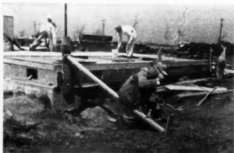
Blocking on the box sill keeps section from sliding off during tilt-up. Alignment of wall and sill is carefully checked.
