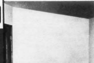
The FIRESTOP wall adjacent to bathroom remains intact and undamaged. On other adjacent walls the intense heat blackened the nailheads, but FIRESTOP Bestwall remained undamaged.
