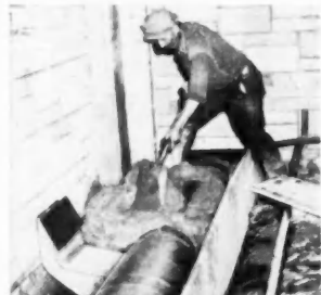
Perlite concrete is poured to 4-inch thickness over pipe in perimeter heating
