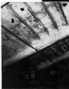
Right photograph shows soffits of concrete seats where concrete has blistered away from reinforcing rods. Rods were sand-blasted and sealed with THORITE Patching Mortar and entire undersurface sealed with THOROSEAL.
