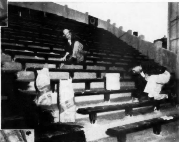
Above photograph shows THOROSEAL FOUNDATION COATING being grouted into upper, or wearing, surface of bleacher seats.
