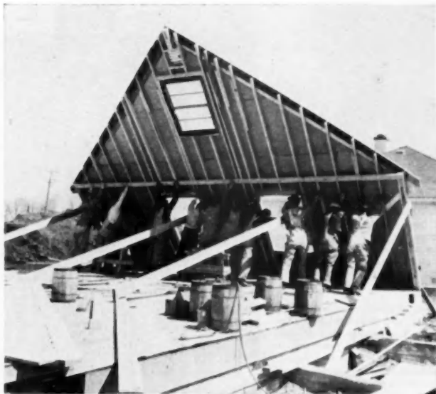
Bracing is pre-nailed to speed anchoring when gable end is in vertical position
