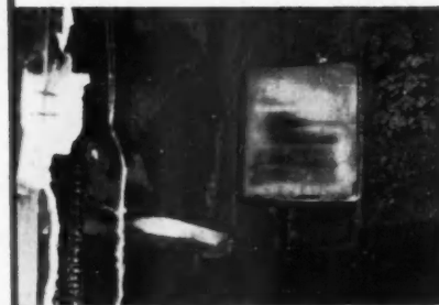
Nowhere has fire broken through the wall, although the tile panels are blistered.
