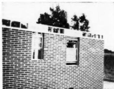
With no six inch lintel available, the builder used a wood lintel. Florida FHA requires a poured reinforced lintel
