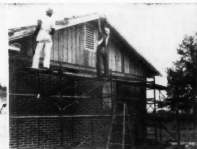
Workmen are trimming out the fly rafter. Note the treatment of the wood lintel after it has been boxed in
