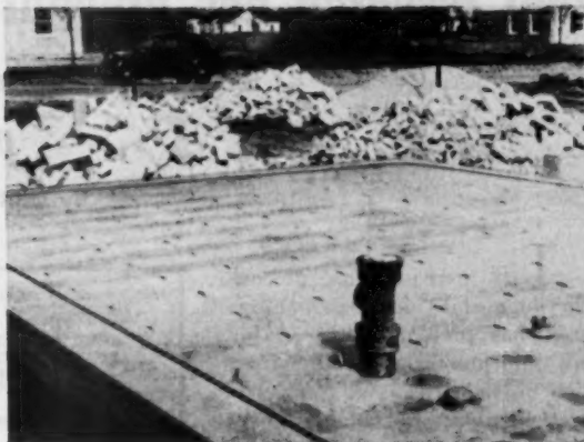
Completed floor slab. Note edge insulation strips and clips for attaching wood sleepers for wood flooring
