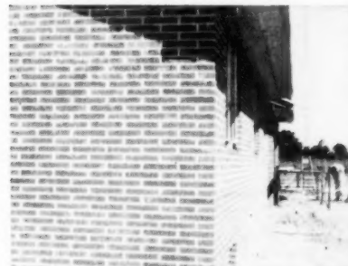
Perfect parallel lines won praise from builder and owner. Builder and masonry contractor remarked at the few culls
