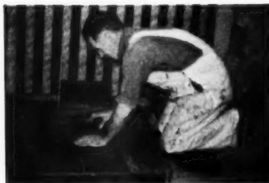
Laying cork tile over impregnated paper cemented to half-inch thick plywood base
