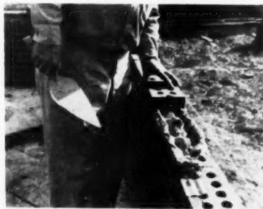
Greater mortar production was found when the mortar was applied to the sides and spread toward the center
