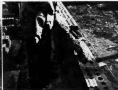
Mason subcontractor found that applying mortar to the center of the brick and spreading to the sides wasted mix
