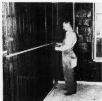
Step 3: Temporary bracing channels are wire-tied to the lath, removed and reused after other side is plastered
