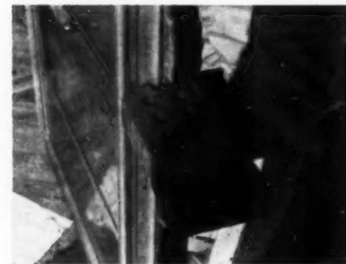
To fit these double hung windows in the jamb slot the corner of the brick had to be cut. Brick is not cut for casements
