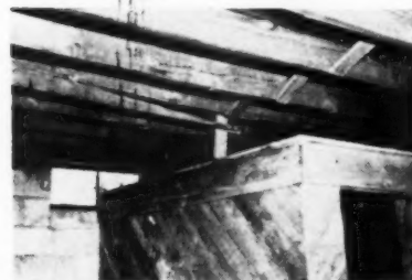
In the basement, beams were cracked
