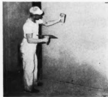
Step 6: Braces are removed to permit plastering to a thickness of two inches. Finish coat is applied and floated smooth chartrain building, but the partition is easily built with a metal base.
