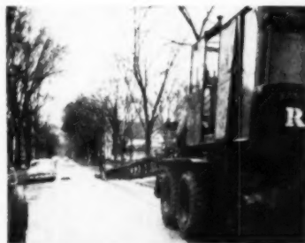
Eighty feet of boom and jib were required to lift the steeple
