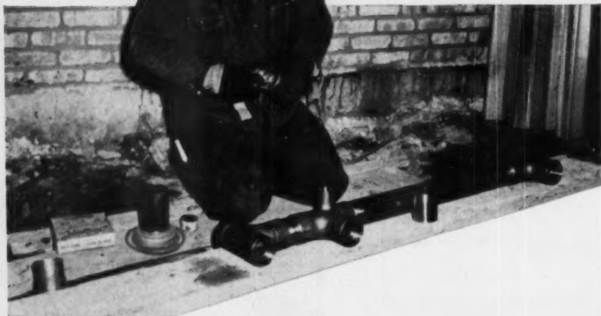
Plumber is polishing joints before fitting assembly together and lifting into position. This prefabrication saves time on the job
