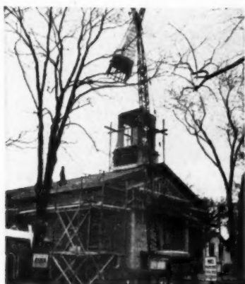
Crane swings steeple over belfry and slowly lowers it into position. Little maneuvering was required to set spire
