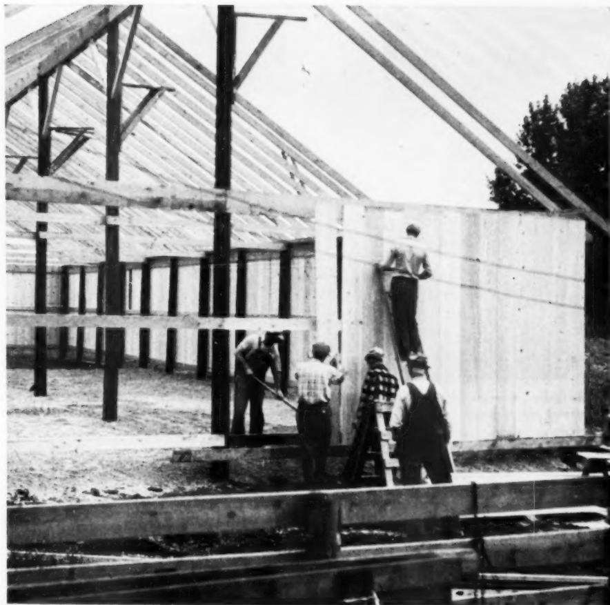
Horizontal nailers located on the posts back up the siding. No battens were used over the joints
