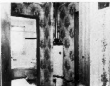
Water heater stands next to plumbing wall in hall. Heat is from wall furnace
