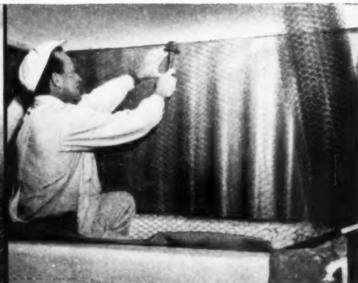
Applying Keymesh reinforcing as a base for interior tile. Notice the ease of handling.
