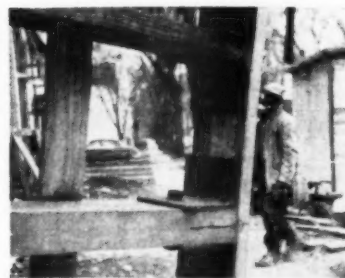
Angle iron brackets are bolted to the belfry and chords of the steeple. Plate below brackets was removed before steeple began its climb
