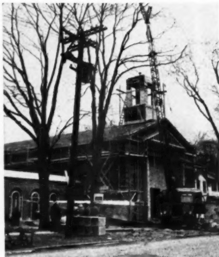
Crane checks close tolerances before hoisting mill-fabricated steeple into place on church top
