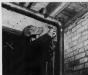
Soldering the copper joint completes operation. Torch heats copper, solder runs into fitting by capillary action
