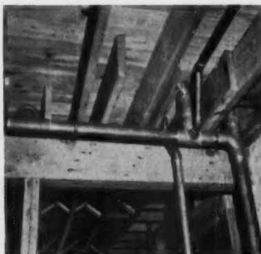
Completed copper assembly for a powder room is shown in this picture
