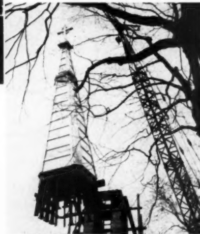
Left cable was attached at three-fourths point and to bottom beam thrust through steeple framework. Line from crane was attached to the upper end. Steeple hung almost straight in its rise
