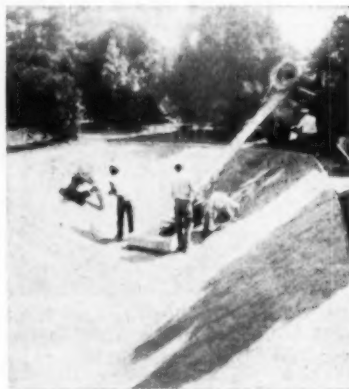
Ready-mix concrete being poured for the two-inch foundation for the pool bottom
