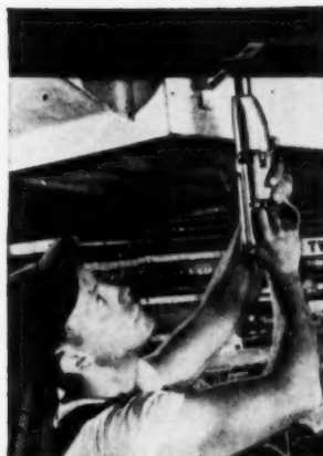
Hanging ventilating duct from concrete ceiling
