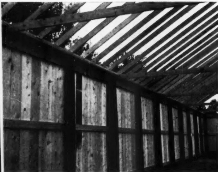
Framing members are nailed to the pressure creosoted poles as support for the skin wall and roof covering
