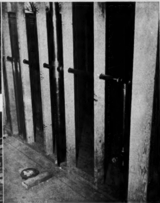
Bathroom installation shows stack and vents. Bath wall is normal 2x4 construction. Pipe sizes are 3-inch stack and 1½-inch waste and vent lines
