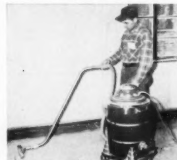
The last step is vacuuming the sanding dust so the floor will be clean for the asphalt tile installation. The vacuum cleaner is also used to clean the house before the buyers take possession
