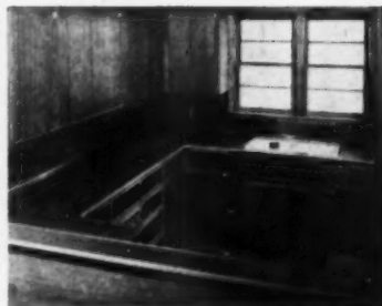
Completed plastic laminate installation. Back splash was installed before cabinets were put up
