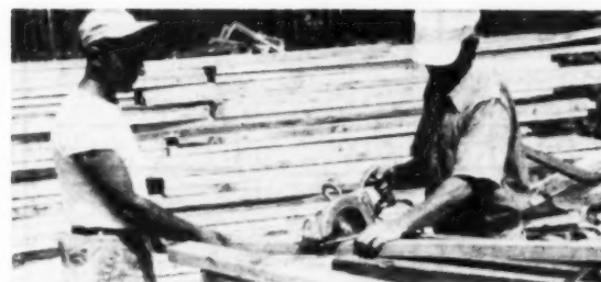
Pattern of truss made to lay out lumber—all cut with an electric hand saw
