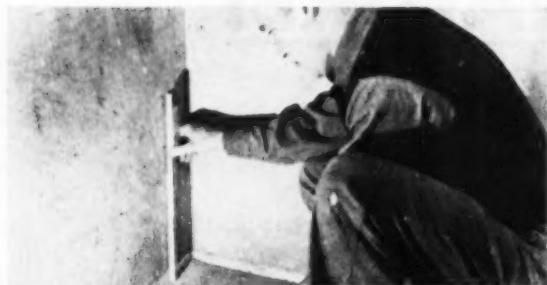
Measuring to obtain leveling point for the application of first course of plastic tile
