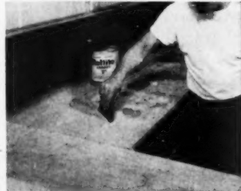
Setting laminate aside, adhesive film is spread over top surface of the installation
