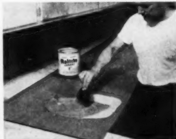
Using applicator furnished with adhesive levels adhesive film on back of laminate
