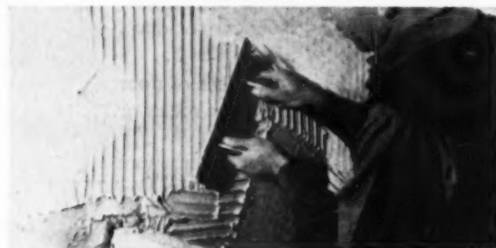
Placing mastic on the wall in diagonal pattern. This will save mastic and permit overall coverage to the plastic wall tile
