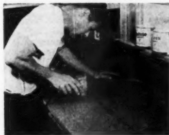
Using Hudee Frame as guide, sink outline is marked; cut out with portable saw
