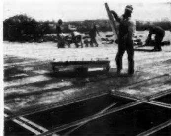
Tectum being applied as roof deck on new Rockwell Manufacturing Co. plant, Uniontown, Pa.
