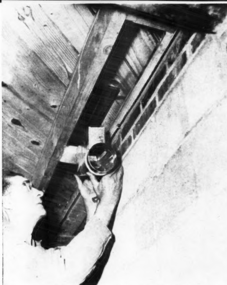
Small pipe duct connection placed in duct spacing, fitted to floor register
