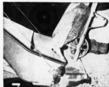
7 Place the dry materials in the skip. Transfer them to the drum while the water is being added. Then mix for at least one minute.
