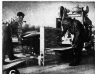
6 Measure aggregates carefully. A platform scale makes for quick and accurate measuring and more uniformity from batch to batch.
