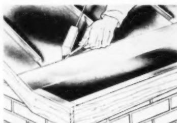
Flat locked seam, with gutter in place, is malletted against roof and soldered
