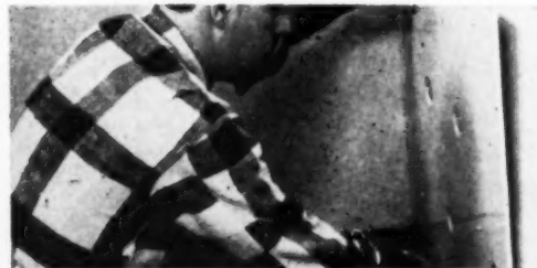
Set end panel in a manner similar to the back panel with the lower edge placed on cardboard tabs imbedded in the waterproof mastic
