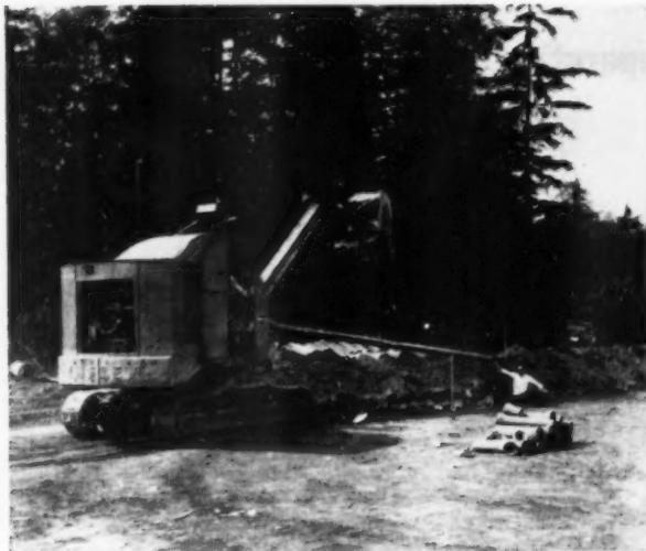
ONE-HALF-YARD UTILITY SHOVEL: most expensive item in Balch's complement of earth-moving equipment, shovel digs sewer and primary water-main trenches
