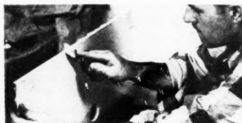
Install end panel in the same manner. Butter the edge which butts against the back panel with pointing compound to insure a waterproof seal
