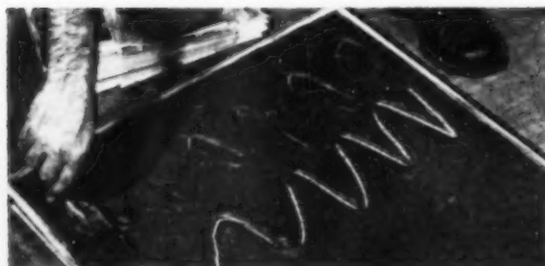
Use a trowel or mastic comb to make serrations in mastic to allow for expansion of mastic when pressure is applied in setting
