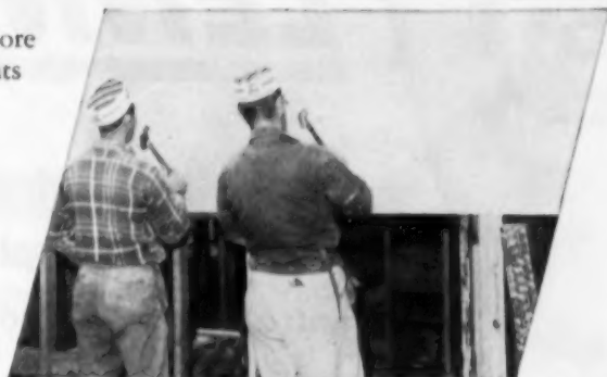
Nailing up Gold Bond Gypsum Wallboard—fast and clean—in a new Cole home in the Dallas area.
