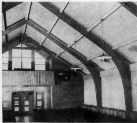
The underside of the roof decking forms the finished ceiling in this small church building. Insulation and acoustical treatment are also provided in this non-combustible roof deck
