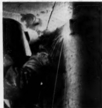
WHEN SLAB HAS REACHED PROPER HEIGHT, steel collars are welded around each column to tie roof and supports together permanently. Work can begin at ground level while jacks are being dismantled and columns are cut flush in preparation for finish roofing
