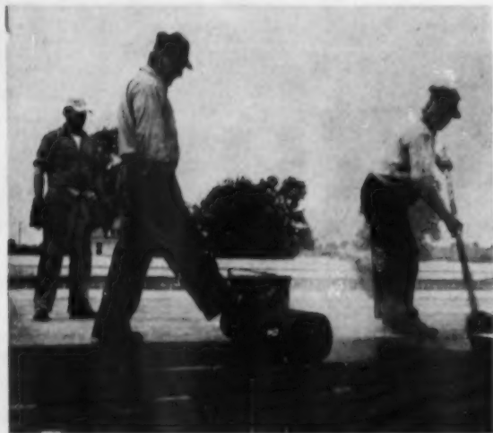
Roofing felts are laid directly to the decking. A factory-applied felt backing eases the built-up roof application and adds another ply to the roof finish
