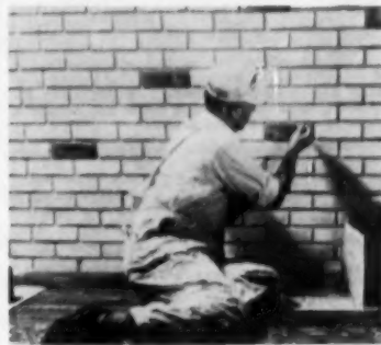
Holl-E-Wood Brick is white in its natural state, is fine base for latex-based paints applied to simulate any of the many natural colors of natural brick. Stiff bristled paste brush is used to paint mortar joints
