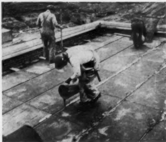
Grout is poured between bulb tees and roof tiles, filling the open spaces. The excess grout is then removed with a plow-shaped device built from 1x6 inch boards. This forms a finish joint
