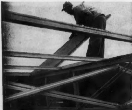
When made in tile form, the material rests on the lower flange of bulb tees which are used as separators for the panels in a steel-constructed roof
