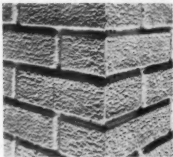
Nail heads and corner are covered with liquid white plastic. Then corner is trimmed with knife, sandpaper or rasp
