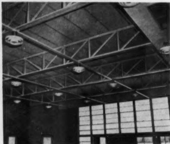
In this school the finished ceiling is the exposed two-inch thick roof tile laid on #200 bulb tees. The exposed ends of the tees are butt welded and the tile grouted on the top side with Pyrofill gypsum concrete
