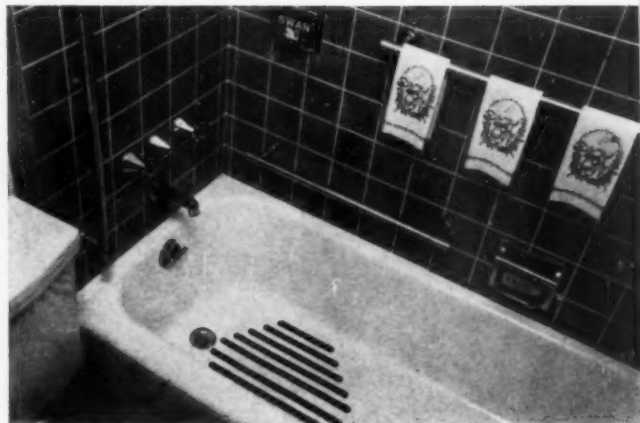
RETIREMENT HOUSE BATHROOM: all rods and soap dishes will support more than 500 pounds. Tub has 1" carborundum strips, variously colored, to prevent slipping.
