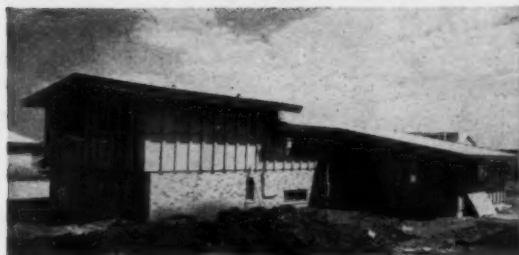
QUINN DESIGNED exterior walls using the Lu-Re-Co system developed by Small Homes Council, designed his panels with horizontal studs to apply Weldwood easier.
