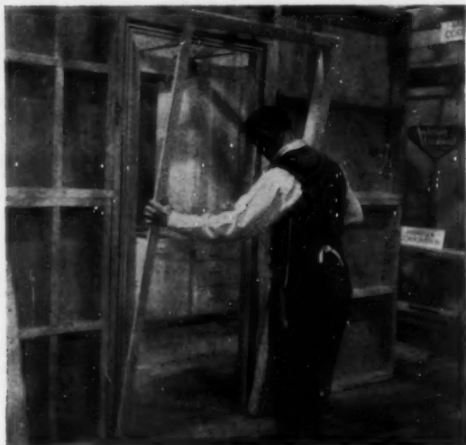
A PRE-HUNG DOOR is set up in the partition. It is merely pushed into place, shimmed, nailed tight, and then the pre-built trim is snapped into place, as shown here.
