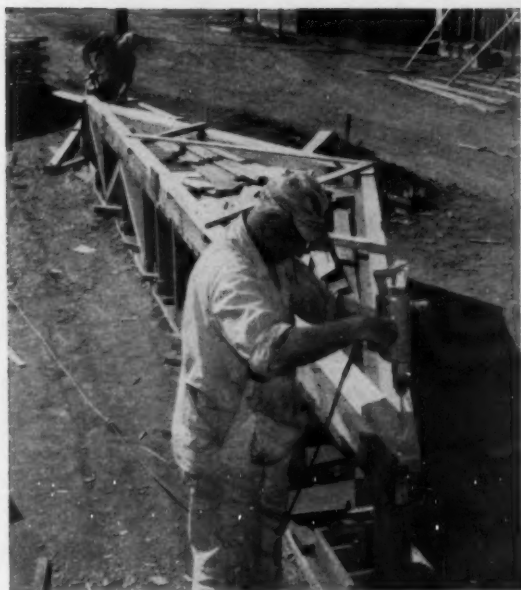
3 SPLIT-RING TRUSS is assembled at the site. All members are precut, so that the building crew does no measuring or cutting, can't make mistakes. A simple jig is all that's necessary for accurate assembly.
