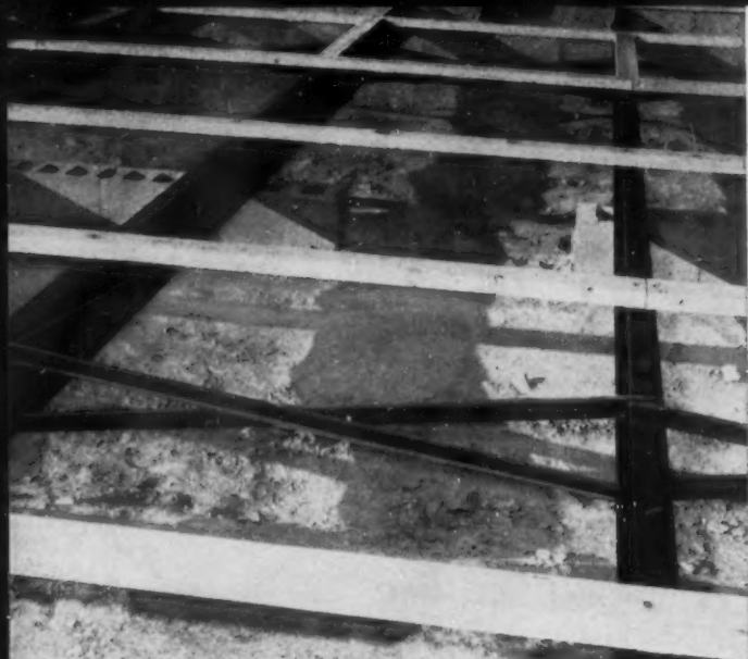
9:00 A.M. Rigid bridging is attached to JUNIOR BEAMS in a continuous row in the center of the 12 foot spans. The 2" x 4"s, laid flat, are securely fastened on four foot centers transverse to the joists.
