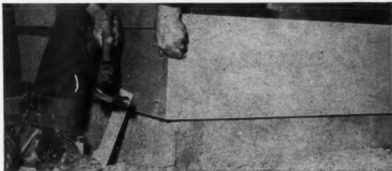
Another Duraply-built home. Corner construction is easy with special aluminum corner pieces that install quickly, cost only pennies.
