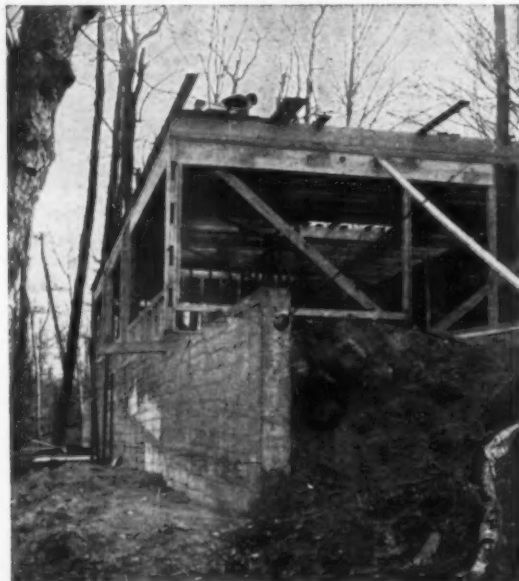
FRONT FOUNDATION WALL is shown during the early stages of construction. Despite the slope, it acts merely as does any normal foundation. The floor slab is tied to it with reinforcing, provides extra front-to-back support.
