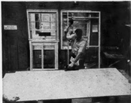
SHEATHING BOARD is stapled on over the insulation. Also used in the demonstration were air-powered, high-speed stapling guns. Any type of sheathing can be used; in this case it is a fiber-board insulating type.
