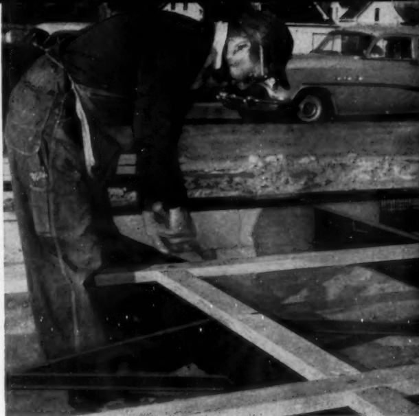
9:15 A.M. In turn, 2" x 4"s are laid along the length of the JUNIOR BEAMS between the transverse 2" x 4"s, providing a four foot grid. A 2" x 6" wood plate is attached to walls to support floor and wall panels.
