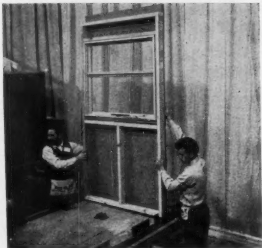
LU-RE-CO WINDOW PANEL is built as a demonstration, and has the window installed. Sheathing overlap is to cover the double 2x6 plate that runs around the house.
