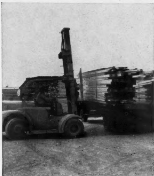
2 FORK LIFT loads a package on truck. Packages are made up ahead of time, so builder gets deliveries at just the right time. Bundles can be dumped off, while panels would require careful, hence costly, handling.
