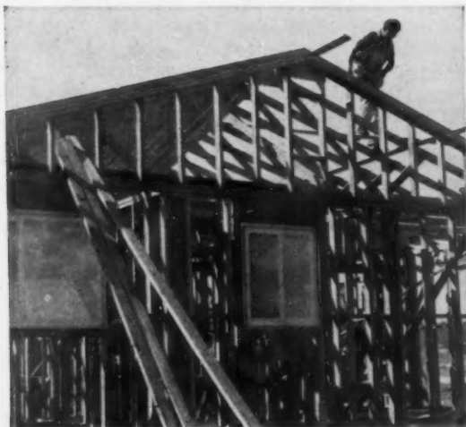
4 FRAMING THE HOUSE becomes a quick, efficient job with precut pieces. Where site work is faster, like the trimming of the sub flooring, it is not done at the lumber yard, instead is left to the building crew.
