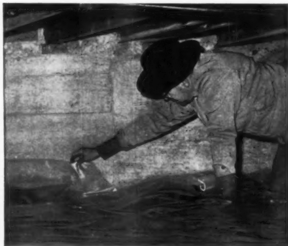
IN CRAWL SPACES—VISQUEEN film banishes musty odors, keeps earth-born moisture away from floor joists.
