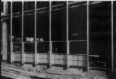
ERECTION begins with sill members to which struts are anchored. Thinlite panels go up vertically on struts.
