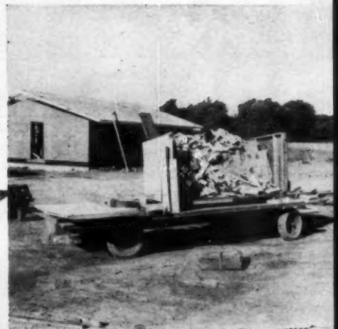
HANDY TRAILER delivers pre-cut bridging to site. Centex makes extensive use of light trailers of various types and sizes.
