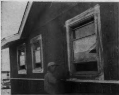
FAST STAPLER is used to tack vapor-proof plastic flashing around windows—a good example of building better with brain power.
