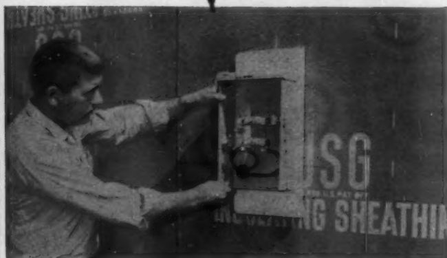
METER BOXES are hung before exterior siding is applied, eliminate need for later cutting and fitting. Centex men are alert for new ideas.
