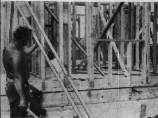
COMPONENTS such as this and the complete window unit behind are built in a nearby yard, delivered for fast and economical erection.
