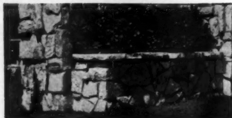
A close-up look at a massive garden wall gives an excellent idea of the rugged beauty given by Palos Verdes "Mossback."
