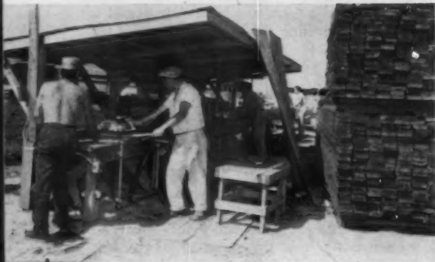
POWER SAW with ingenious home-made rig saves $1,000 a week in rafter cutting and notching. Centex stresses precutting, components, know how.
