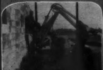
Davis Backhoe on Work Bull 202 digs flush alongside obstructions, lets you load directly into trucks.
