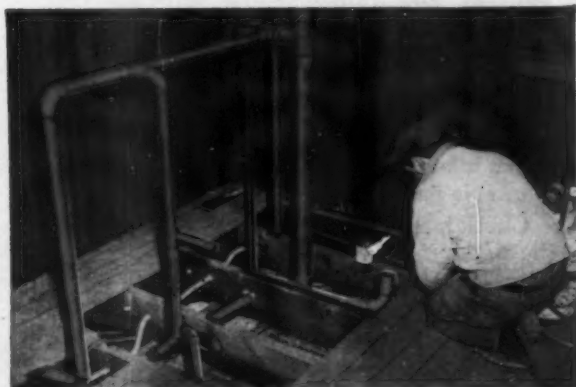
ROUGHING-IN for a bathroom on the third floor. Note small area of flooring removed—also that only small holes were needed in the old floor joists to install the copper tube waste line.
