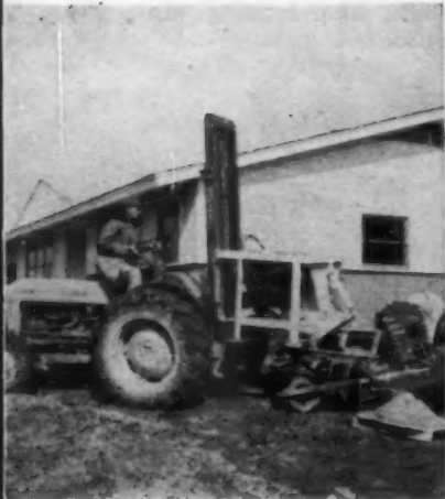
IN HEAVY MUD , fork-lift tractor delivers bucket of concrete direct to wheelbarrow at site.
