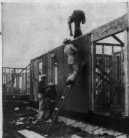
SPECIALIZATION cuts costs. This crew of four sheathes about five houses a day. Crews move in and out fast, are expert at each operation.
