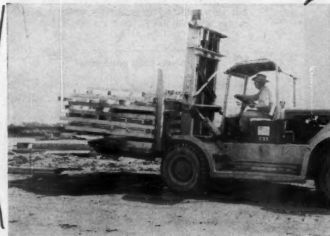
FORK LIFT truck speedily delivers pile of wall components to site, spots them exactly where needed. Most materials are palletized for easier handling.
