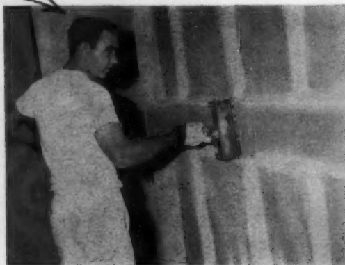
SPECIAL smooth-on device speeds up plastering of dry-wall joints, does a better job. Each building operation is highly specialized.
