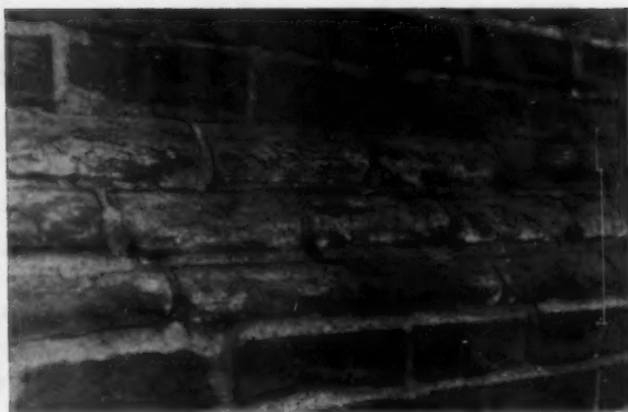
SPALLING AND EROSION resulting from moisture penetration
