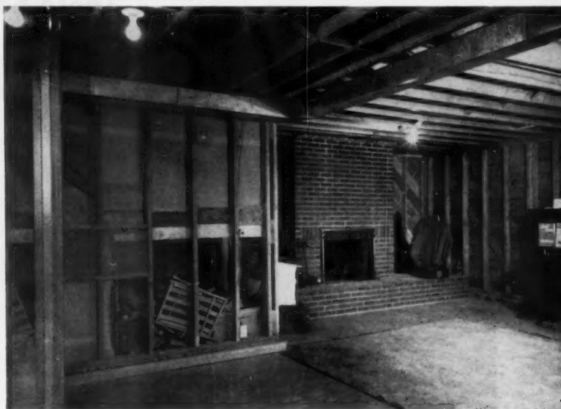
PORTIONS OF CHILDREN'S PLAY area and adult area as they originally appeared. Builder Knut Haga of Seattle did the work. He says the job has had a promotional effect, has led to many similar remodeling projects.
