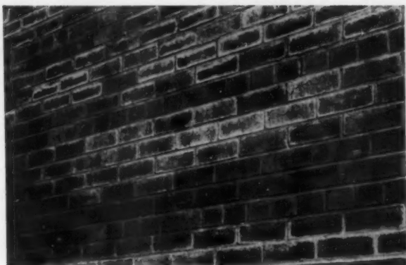
EFFLORESCENCE causes white stains as water penetrates masonry
