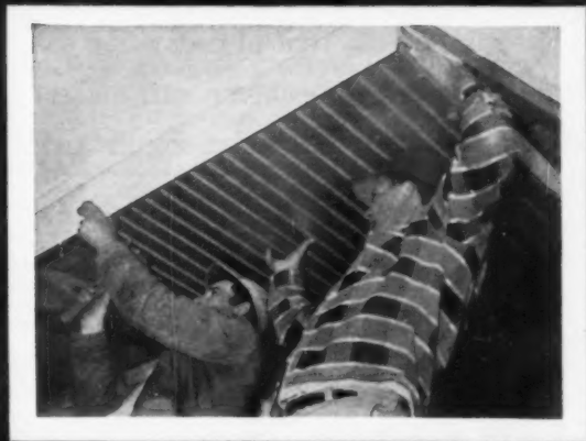
ALUMINUM SOFFIT, also experimental, is nailed at wall and fascia. Ribbed construction requires no outlookers.
