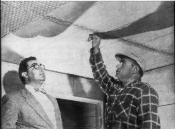
Eby (left) inspects application of Keycorner, used to reinforce joints. Keycorner is also used at all wall and corner junctures.
