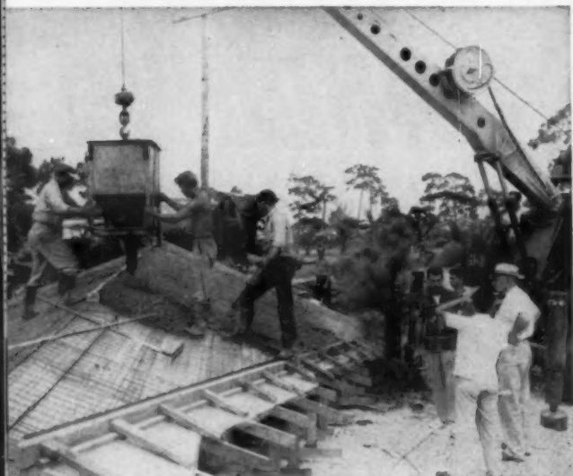
EIGHT SECTIONS of this folded-plate concrete roof were cast in layers—four to a form, separated by Visqueen polyethylene film. Seven-bag mix was used. Lightweight aggregates helped minimize weight of the roof.
