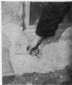
In basement cracks
