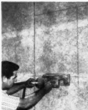
Wall sections are set solid and openings are cut out with Skilsaw quickly and easily.
