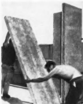
Tilt-up wall construction technique for fast wall assembly with only two men.
