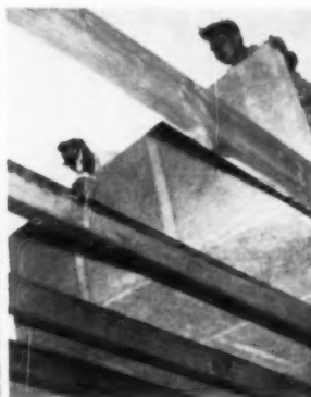
High insulating Cemex panels sheath roof quickly and acoustical ceiling is "free."
