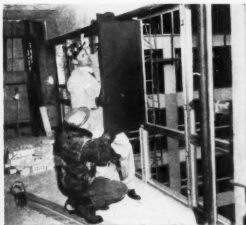
▲ INSIDE WORK —Workmen fit U.S. Plywood's Weldwood panel into grid from inside building. This saves cost of scaffolding, common to curtain-walls.
