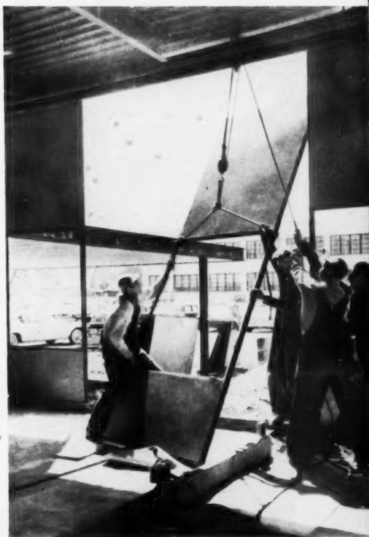
▲ PORCELAIN FACE —Fiber glass insulates core of porcelain-faced steel curtain-wall panel. Workmen position it with tackle temporarily mounted to beam.
