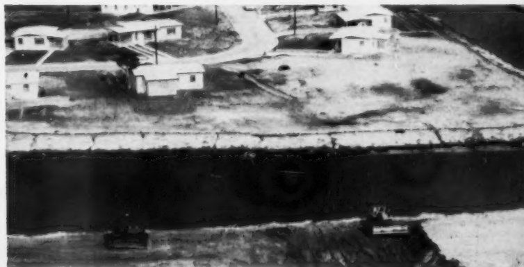
FEED DOZERS —Caterpillar tractors fitted with dozer blades build fill to elevation of 4½ ft. Dozers also slope canal banks, later sod them.
