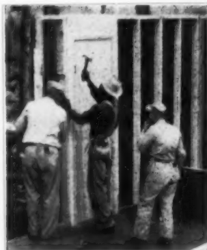
Big parts like these wall panels, used instead of small pieces, speed the work of framing crews. ▶
