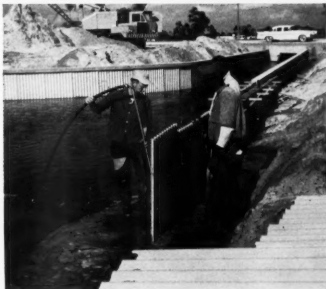
NEW BULKHEADING —Workmen water-jet National Gypsum's corrugated transite bulkheads into place along canal banks. Panels, impervious to marine borers and rot, are anchored by cable to concrete deadmen.
