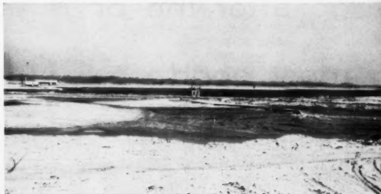
HELPS DREDGE —Huge dredge opens main canal and hydraulically moves fill ashore. Dredge, with dragline, handles 1,500 yds. daily.
