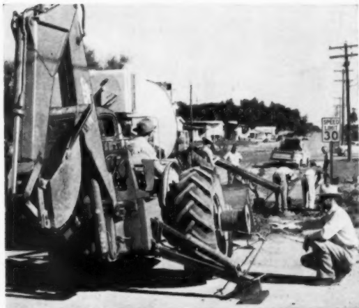
HOMEMADE WINCH —Contractor Tague jacks up one end of his Ford Model 1800 pneumatic tractor by extending its digger stabilizer foot alongside one wheel. Fitting a drum with cable to the wheel creates an effective, controllable winch that holds a sufficient cable length.
