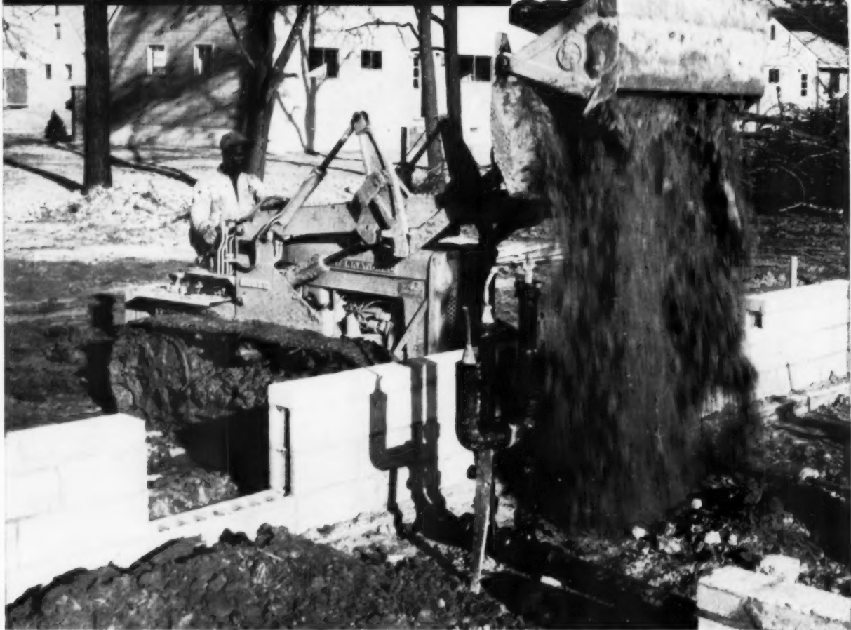
INTERNATIONAL-HARVESTER'S T-340 crawler with Drott's 4-in-1 bucket clamshells fill into basement of house at
