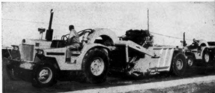
LOADING —Adjustable belt loader fitted to bow of scraper bowl eats into sub-base. Belt then loads dirt into bowl without push-tractor help.
