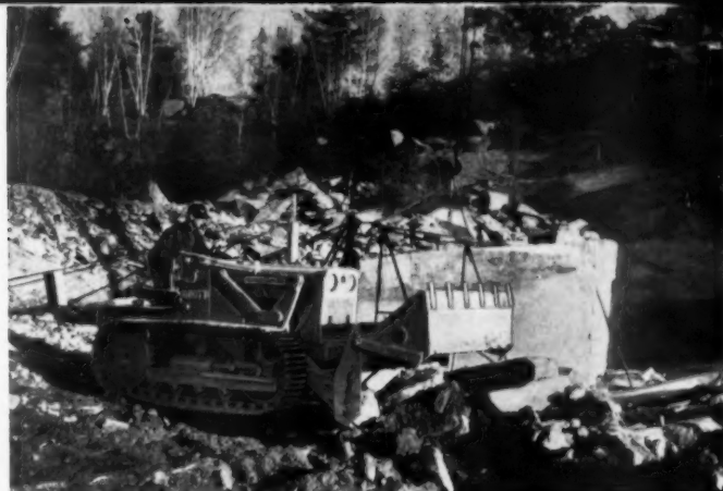
Dozer moldboard is tilted forward or backward to increase or decrease depth of cut for precision grading accuracy.
