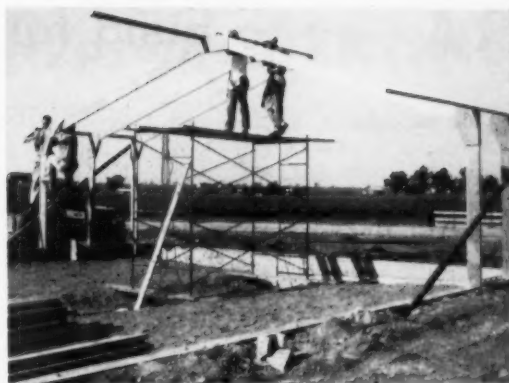
4 COMPLETED FRAMES are put into position after field-applied glue has cured. Here, nailers and bracing are being applied to hold the frames in position.
