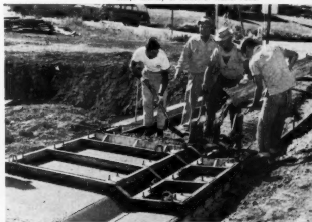
PULLS HOMEMADE SCREED —Curb and sidewalk screed, fabricated from sections of channel steel, rides over steel forms. Screed both strikes off concrete at proper grade and rough floats the surface. Tractor screed team cuts labor by 60 per cent over previous hand methods.
