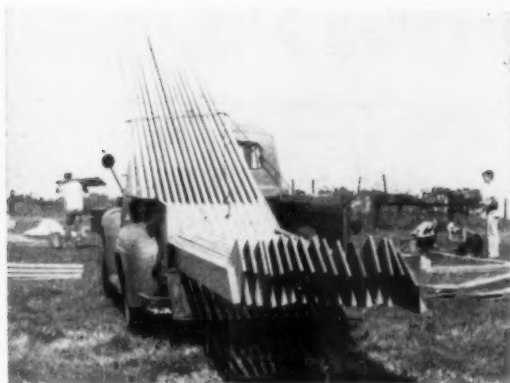
3 HALF-FRAMES —following a 24-hour curing period at 70° F.—are delivered to the site for final assembly. The ones shown here will span 30'.
