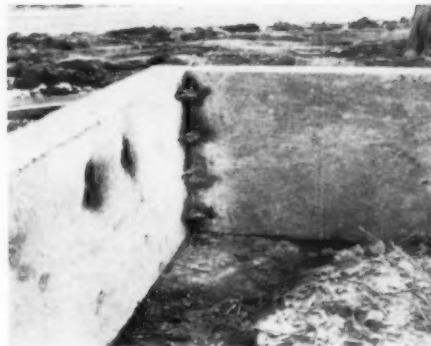
REINFORCING BARS are cast into beams and piers. When beams are set, rods are hammered tight together, fastened permanently with arc welder.
