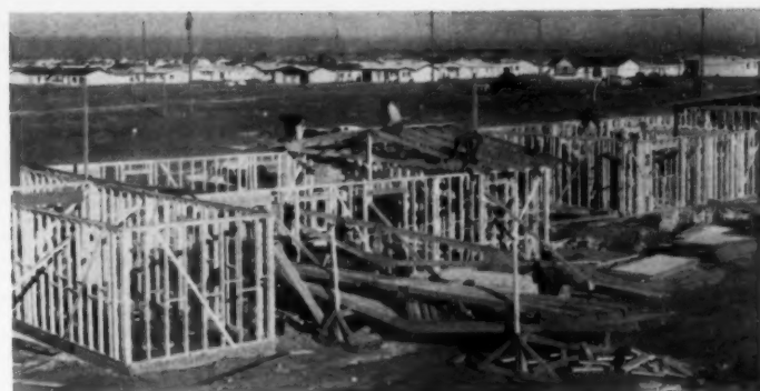
MOVABILITY —Specially-designed trailer (top photo) takes trusses, 3 men, to house site. Bottom, 3 carpenters meet them. Team finishes assembly in 1 hr.
