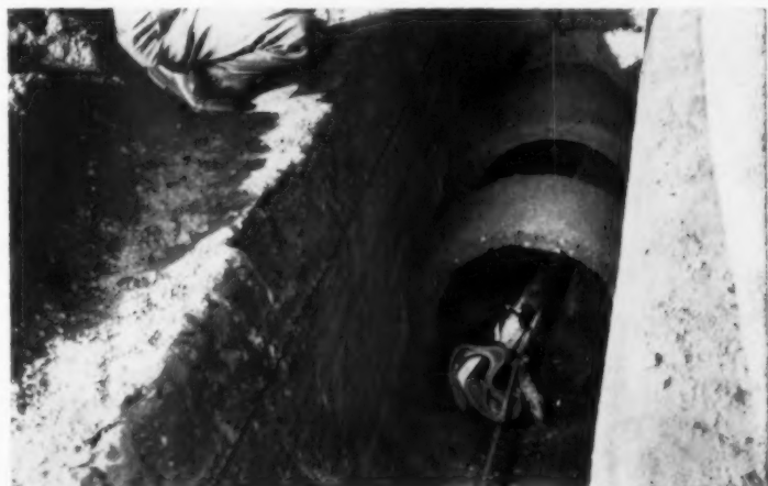
CORD EXTRACTS TUBING —Once concrete has set the inner form is then deflated. A nylon rope attached to grader blade pulls it free from concrete pipe. Patented process belongs to Fullerform Continuous Pipe Corp., Phoenix.
