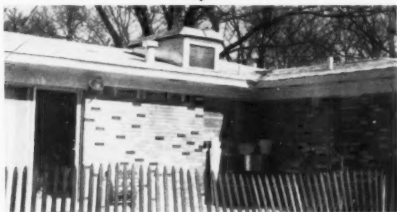
REAR VIEW of new-home installation. Prefabbed gable is mounted on rear pitch of roof to house central cooling unit.
