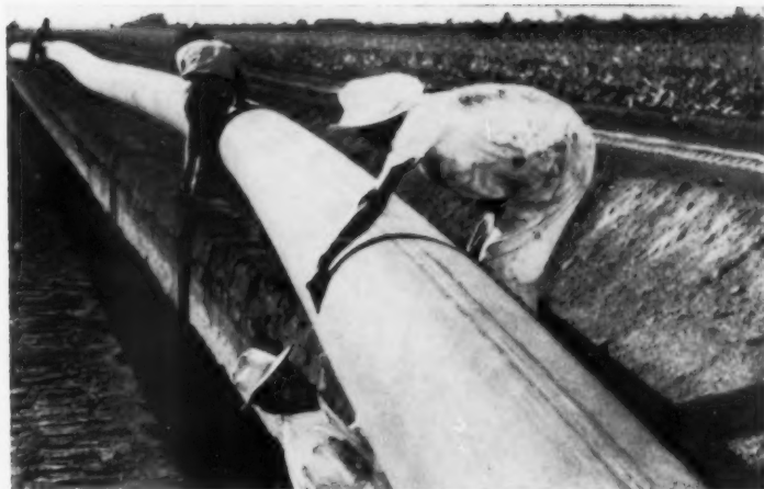
WORKMEN PLACE FORM —Inflatable rubber and fabric hose-like concrete form is lowered into freshly dug trench. Designed by Aircraft engineers, the inflatable form shapes the inside of the pipe for runs of 300 ft. in length.
