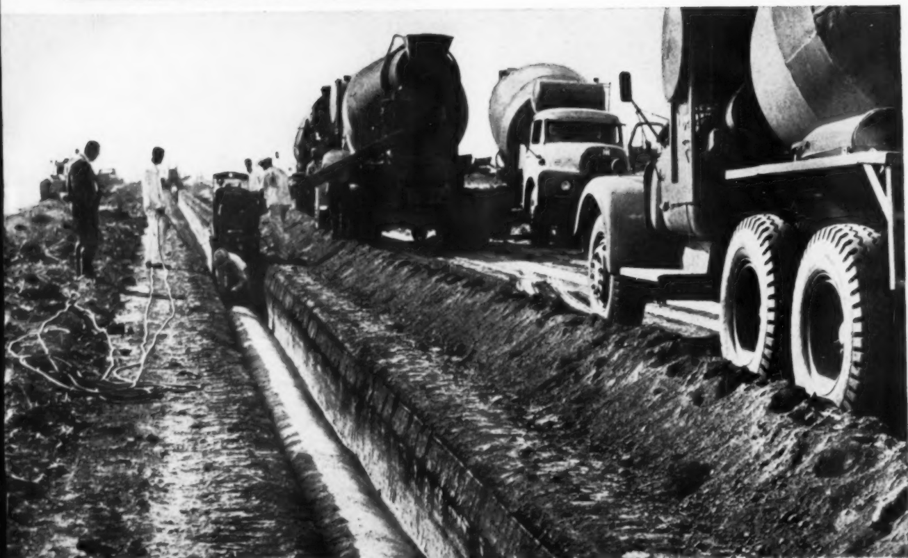
TRANSIT MIX TRUCKS move swiftly alongside freshly cut trench and pour concrete over unique forming device that lays
