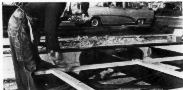
FASTENING SLEEPERS —Crew first nails 2x4's on 4-ft. centers at right angles to beams. Sleepers go in between, then are fastened to the beams. Non-adjustable rigid bridging is used between the beams.
