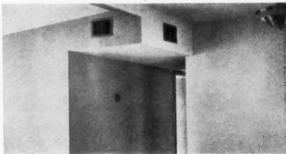
COOLED AIR is discharged into rooms from small ducts shooting off from central duct housed in drop hallway ceiling.
