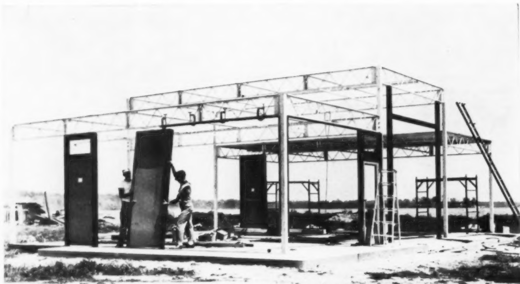
PUT UP WHOLE BUILDINGS —Macomber's "V-Lok" service station in Bridgeville, Del. Designed by American Metalcore Systems, this building goes up in a week.
