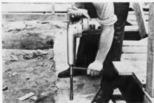
DRILLING of foundation holes to bolt down the house frame is easy for this electric hammer with star drill.
