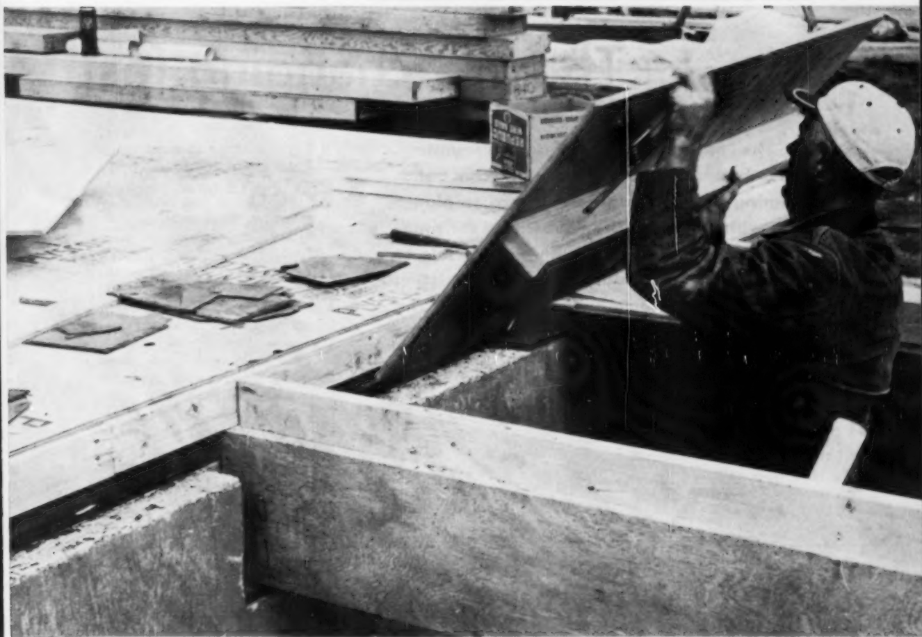
2,000-SQ. FT. FLOOR SYSTEM , including subfloor, can be laid in under six man-hours with Douglas Fir Plywood
