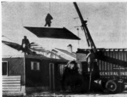
COMPACT folding boom extends 40 ft. in air, lifts component panel for roof into place in one smooth operation.
