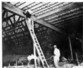
Construction work continues without interruption. Aldrin chemical control of termites eliminates costly shields, makes application easy.
