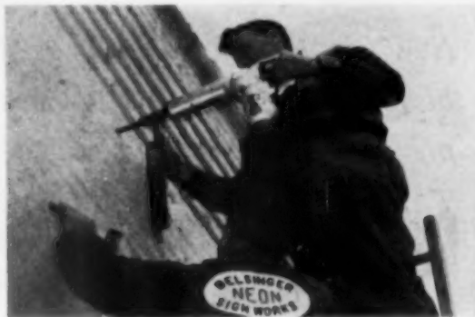
PIERCING of brick wall for sign hangers is accomplished by Black & Decker electric hammer with star drill.
