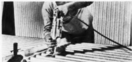
POWER-PACKED Milwaukee hacksaw cuts corrugated aluminum, makes intricate cuts for fitting around pipes.
