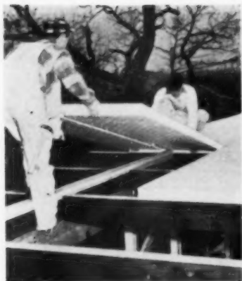
ROOF PANELS were nailed down with 40-d nails. This edge panel was dadoed to reduce heat loss.
