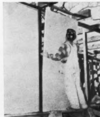
BUTANE-TYPE caulking tape went on before installation of outside stops. Closing-in took two days.
