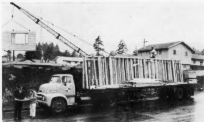
ERECTION SERVICE comes complete with four-man crew. Crew does foundation work in two days including floor; completes framing in a week.
