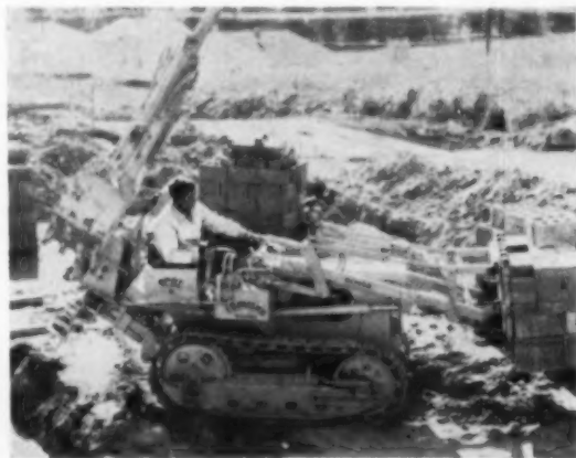
CRAWLER TRACTOR with fork-lift attachment transports big load of concrete blocks, frees men for other jobs.
