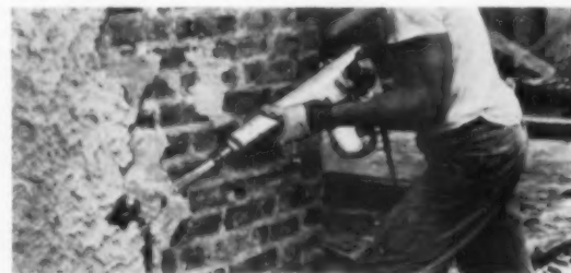
PORTABLE electric hammer with chisel attachment enables this workman to remove old stucco much faster.
