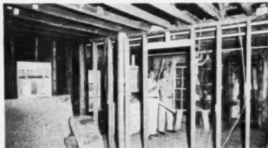
INSIDE REMODELING of Burns & Wisner's old house. It will include new wiring, plumbing and wall finishes. Only outside walls will be left untouched.
