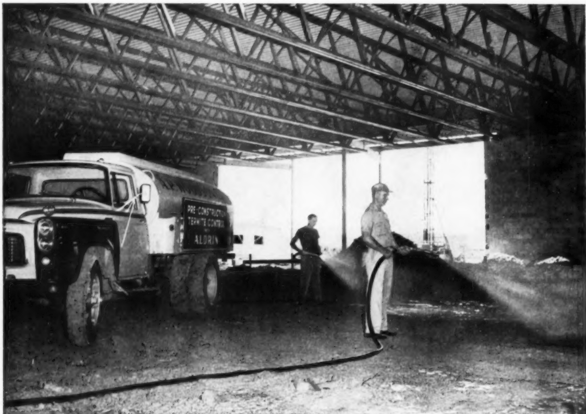
No wood-eaters here. A. P. Woodson Co. "termite-proofs" the Springfield Bowling Lanes (40 lanes) with aldrin termite control.
