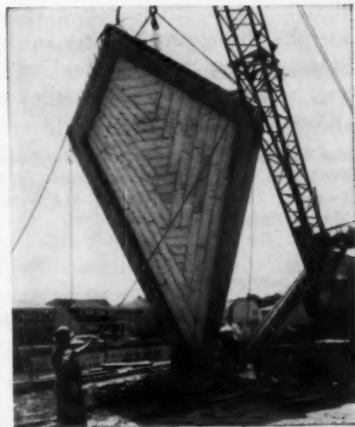
1 1/2-inch Styrofoam serves as form liner, permanent insulation and base for plaster in this lightweight tilt-up panel.
