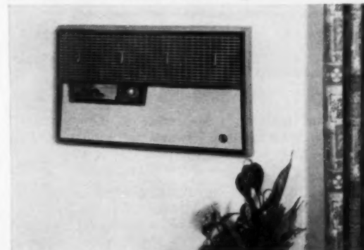
ONE-THIRD OF THE LESSEES arranged to have through-the-wall air conditioning by Westinghouse . . . offered optionally . . . to assure hot-weather comfort.
