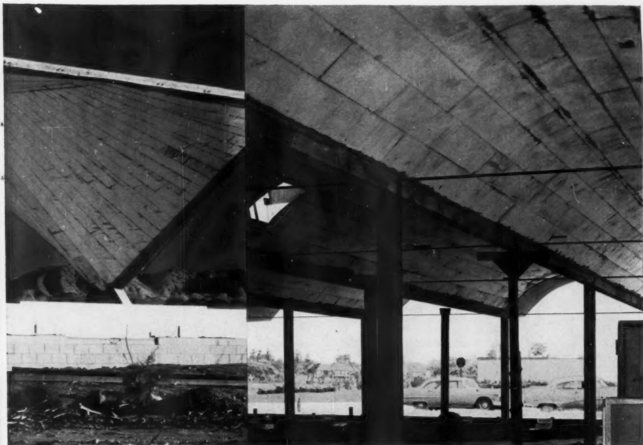
Hyperbolic paraboloid (above) and barrel-vault roof (right) show Styrofoam insulation form liner ready for plastering.
