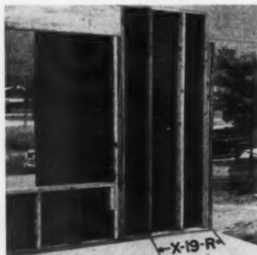
Panel 19-R (see blueprint) goes up first. Framing is on 16" centers. Panel is cut down to receive carport beam. One piece of sheathing, 32" wide was used here.
