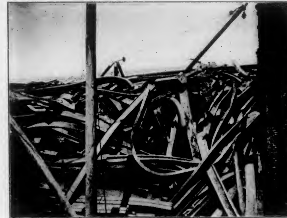
Fig. 1. Showing Bent and Twisted Steel Taken From the Old Emporium Building
