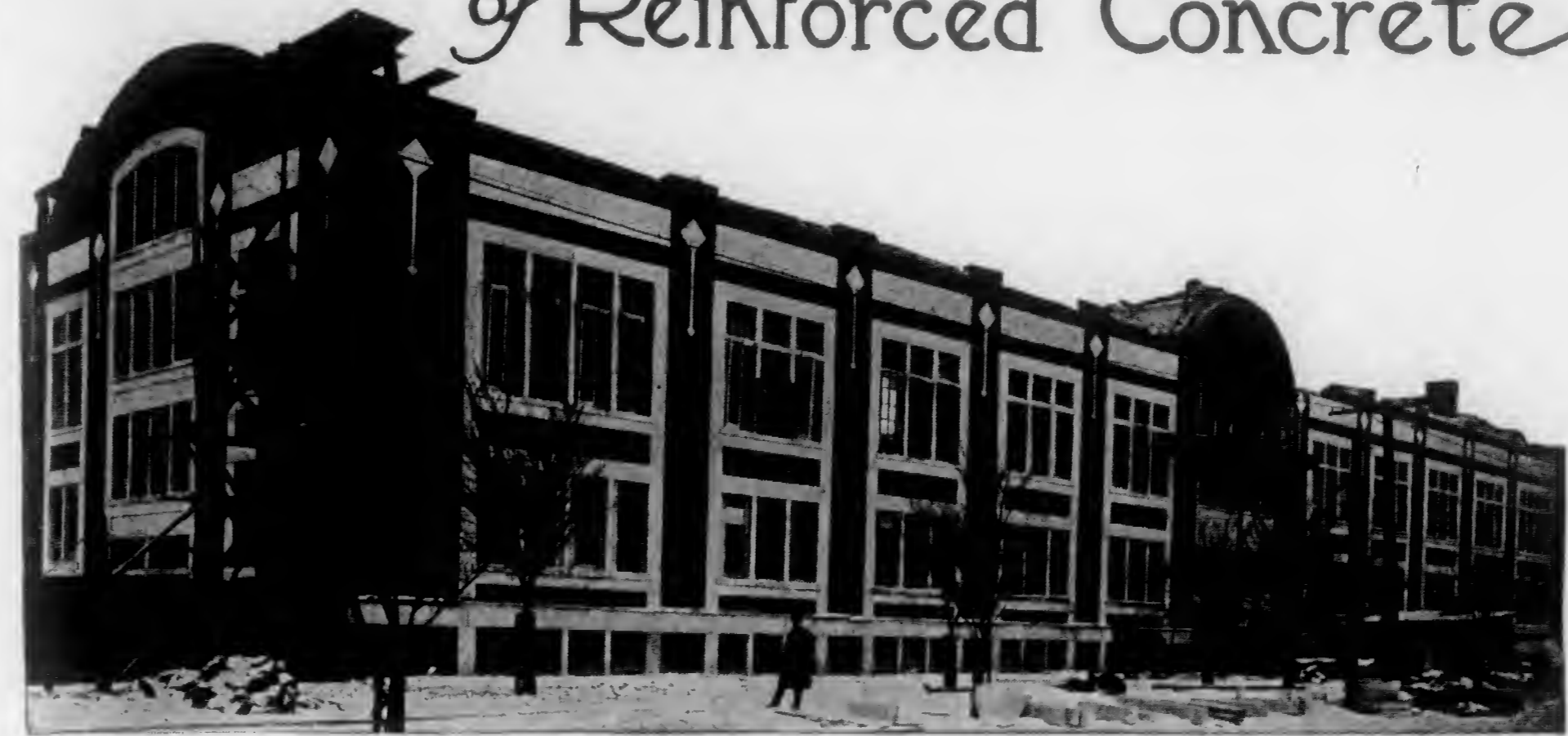
The Administration Building of the Geo. N. Pierce Manufacturing Plant at Buffalo taken during the process of construction. This immense plant, having over 325,000 square feet of floor space, was built throughout according to the Kahn System of Reinforced Concrete.
