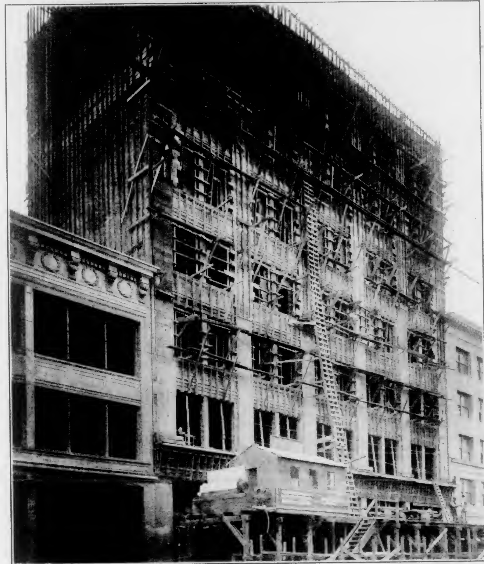
The Macdonough Building, San Francisco View From Kearny Street, Taken Four Months After Excavation Was Begun; Note That Five Sets of Forms Are Used
