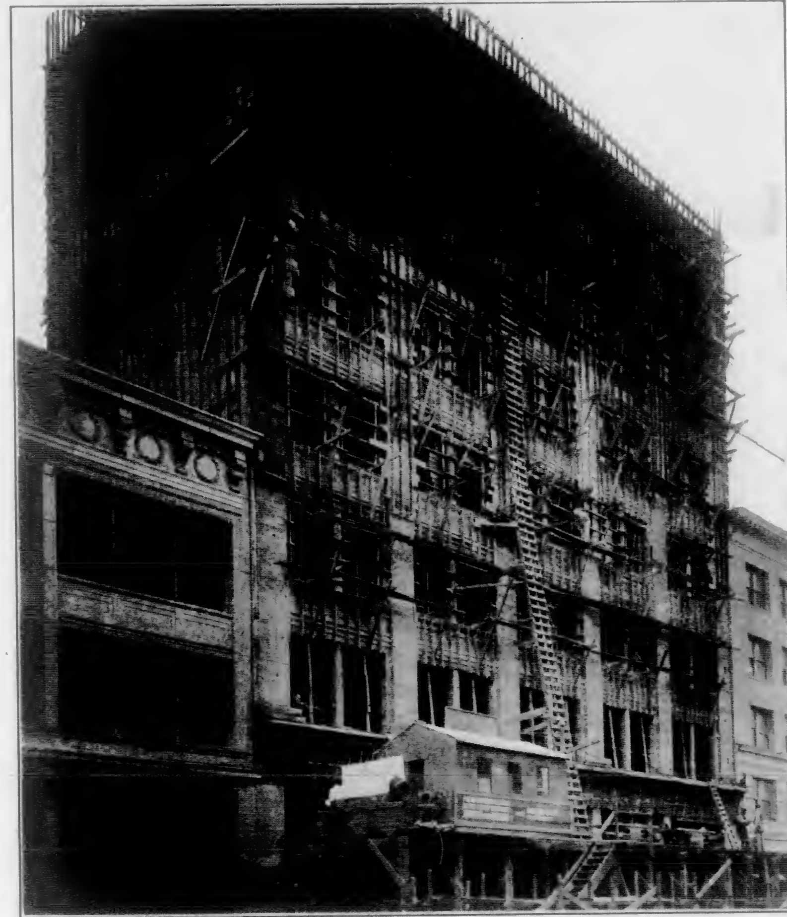
The Macdonough Building, San Francisco View From Kearny Street, Taken Four Months After Excavation Was Begun; Note That Five Sets of Forms Are Used
