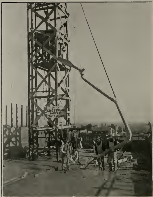
John Luckenbach Office and Loft Building, Los Angeles, California Edelman & Barnett, Architects Showing Tower and Pipe Line for Pouring Concrete
