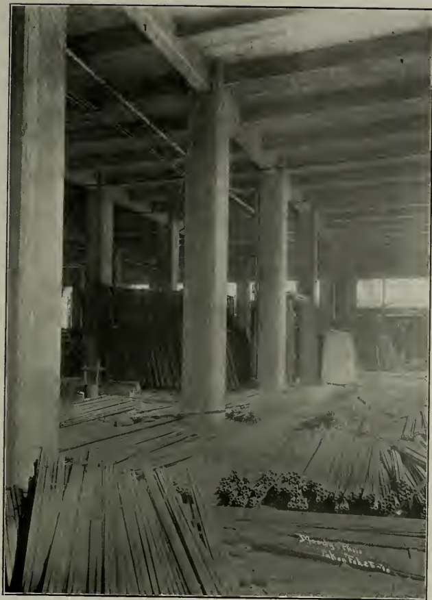
Photo of First Floor After Removal of Forms, Showing Slab and Beam Systems of Construction. A. L. Haley, Architect
