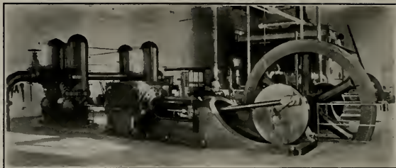
One of the Engines, Power Plant Thomas Higgins Building, Los Angeles
