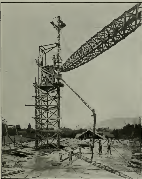
First Church of Christ, Scientist, Pasadena, California Franklin P. Burnham, Architect Showing Gravity System Triangle Tower Used with Boom, and Single Pipe Line
