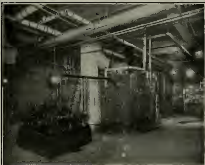
Hotel Sacramento. Boiler Room
