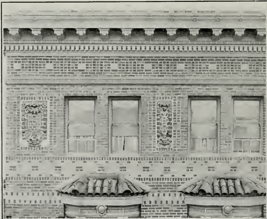
Detail of Top Story of Schmiedell Apartment House, San Francisco, Fred H. Meyer, Architect Showing Rustic Pattern Brick Work and Terra Cotta Panels as Executed by N. Clark and Sons
