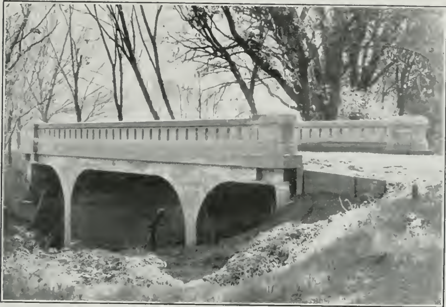
Reinforce Concrete Flat Slab Bridge, City of Ross, Marin County, California John B. Leonard, Engineer
