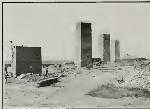
Showing Forty Foot Stacks of the Pacific Sewer Pipe Company's New Plant under Construction at Los Nietos
