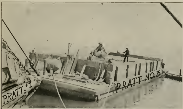
Unloading part of a 5,000 yard (equal to 200 car loads) order of washed gravel with clamshell bucket at Bolinas Bay for the J. G. White Engineering Corporation
