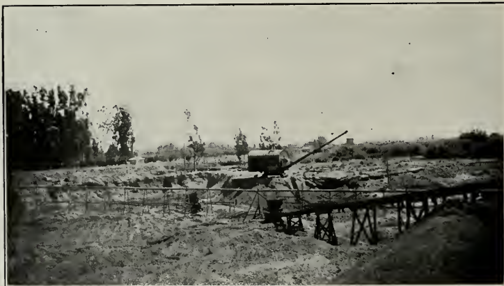
Panoramic View of Gravel Beds, Electric Elevator, Plant and Locomotive Crane of the Niles Sand, Capacity 1500 Yards
