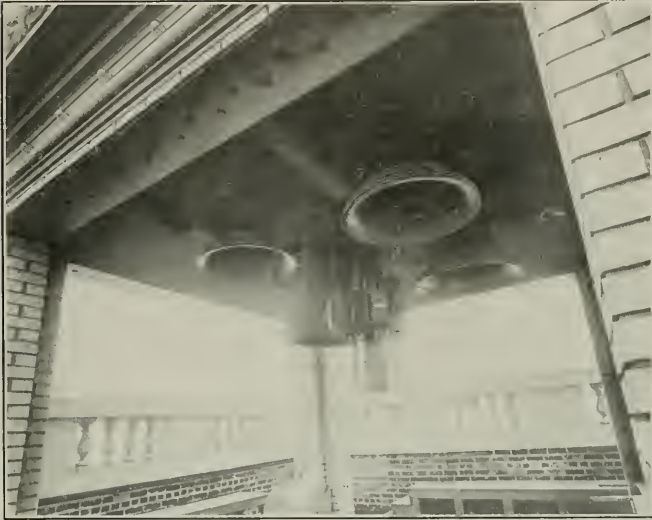
Electrically Operated Westminster Chime of Bells Installed in Tower of Oregon Journal Building, Portland Oregon, by THE STANDARD ELECTRIC TIME CO.
