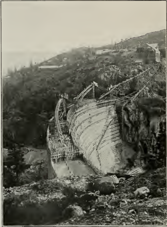
Birds'-Eye View of the Spaulding Dam Four No. 14 Smith Mixers and Two Clyde Cableways used
