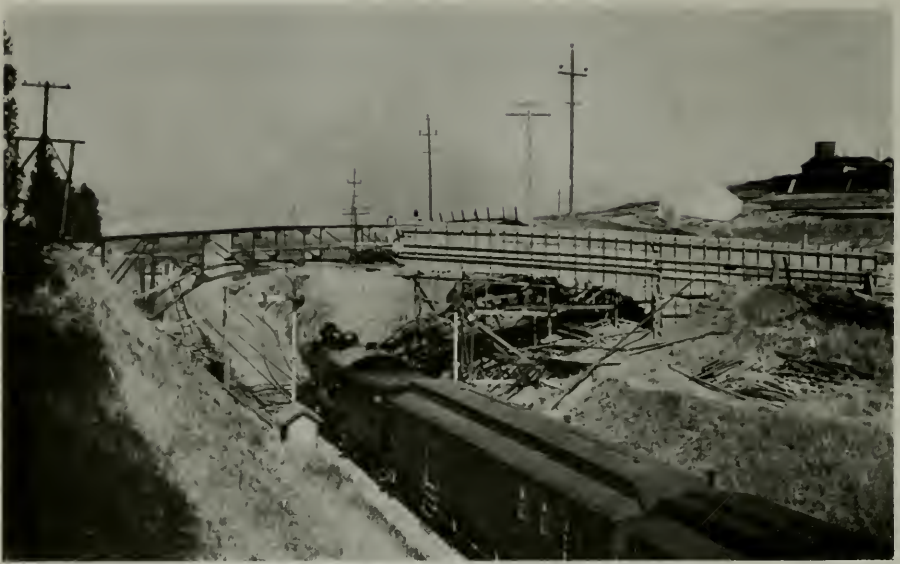
PROGRESS VIEW, CANTCRETE BRIDGE OVER SOUTHERN PACIFIC TRACKS, PEYTON, CONTRA COSTA COUNTY.
