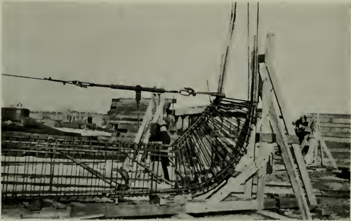
FIG. 4—Bottom frame steel of the Atlantis, built up as a unit on the ground and by means of a cable and ratchet pulled together at top to facilitate placing frame inside the shell steel previously erected.
