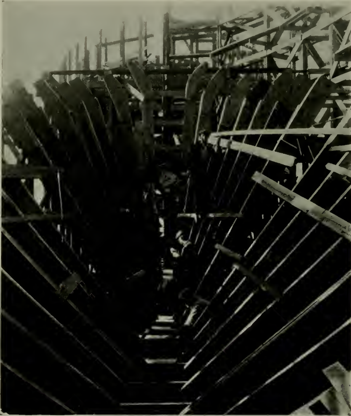
LOOKING AFT IN 7500-TON CONCRETE OIL TANKER, SHOWING STERN FRAME IN PLACE
