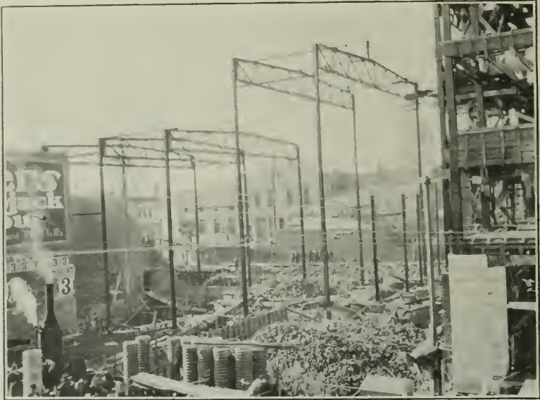
These columns and trusses were put up for a moving picture house without lateral and sway bracing. It was difficult to keep the members plumb with cables and dangerous to the men working 60 feet above the ground without any planking or safety nets below them.
