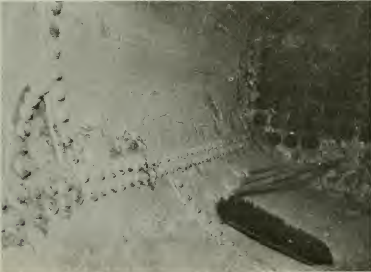
THREE-EIGHTHS INCH PLATE EATEN AWAY ALMOST ENTIRE LENGTH OF BOILER
