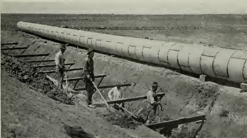
FORTY-EIGHT INCH ARMCO PIPE BEING INSTALLED IN IRRIGATION DITCH, RECLAMATION DISTRICT NO. 1500
