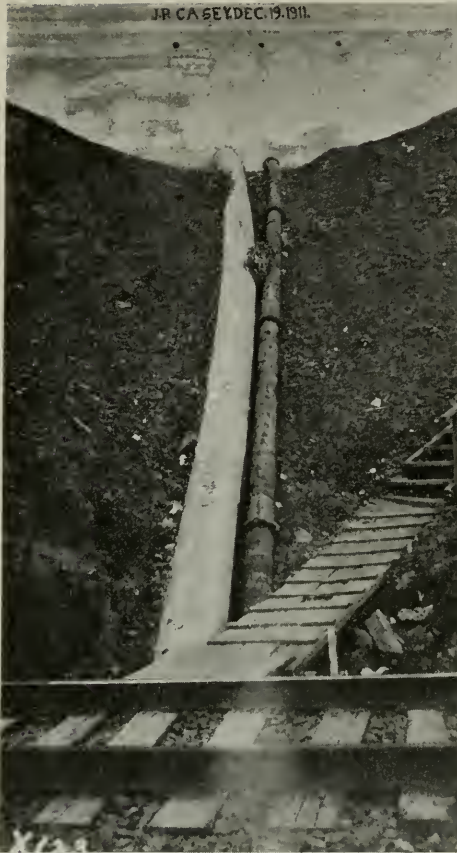
Armo corrugated pipe leading from concrete wall at edge of highway underneath railroad tracks.
