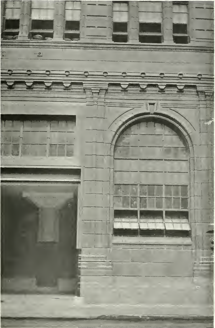
DETAIL AT SHIPPING DEPARTMENT, BUILDING FOR THEO. H. DAVIES & CO., LTD. HONOLULU, T. H. LOUIS CHRISTIAN MULLGARDT, ARCHITECT Terra Cotta manufactured and erected by Gladding, McBean & Co., San Francisco.
