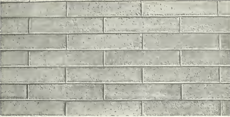
Section of STONE-TILE wall showing colored mortar joint markings and texture of brick surface
