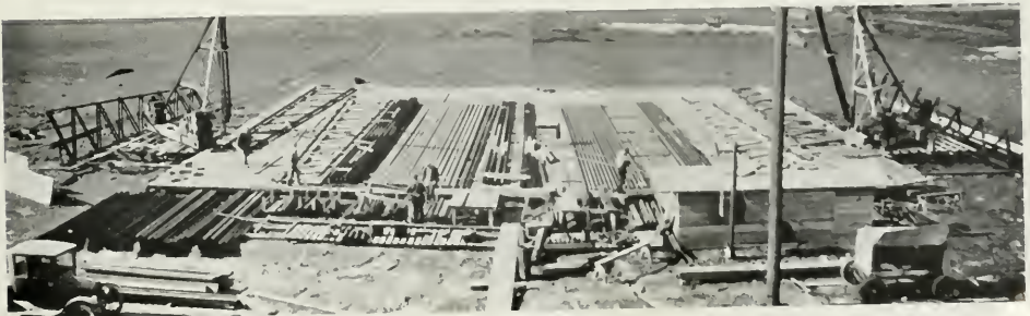
WELDING PLATFORM AND STOCK PILES, A STRUCTURAL ENGINEER ACTING AS FOREMAN. FOUR WELDERS AND TWO LABORERS FABRICATED FIVE TRUSSES PER DAY
