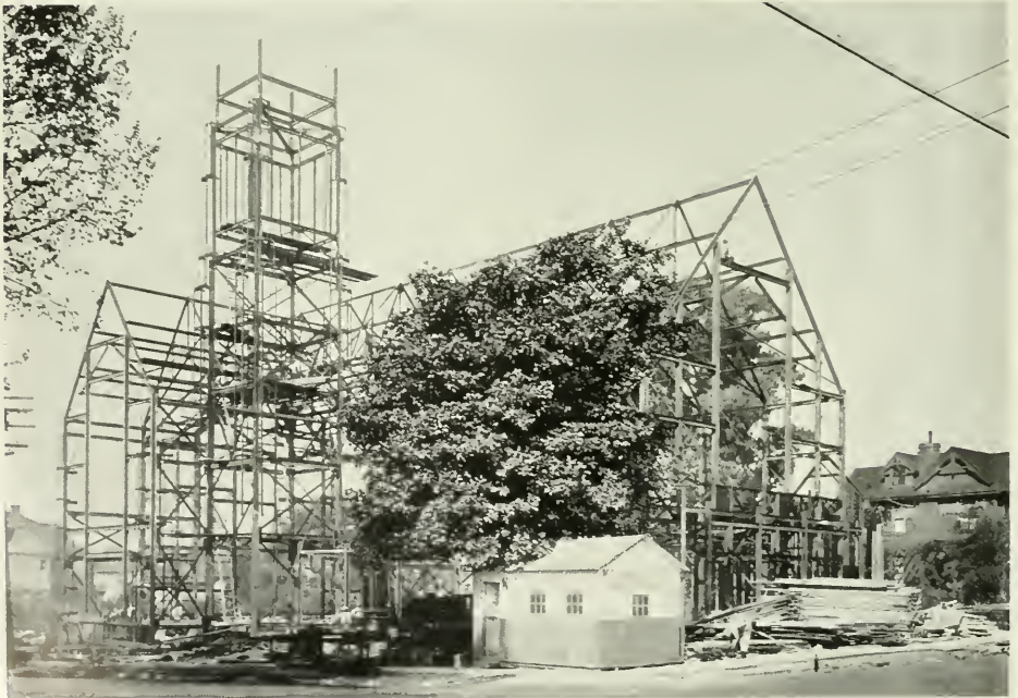
Structural Steel Fabricated and Erected by Pacific Coast Engineering Company FRAME OF FIRST METHODIST CHURCH, BERKELEY Henry Dewell, Structural Engineer
