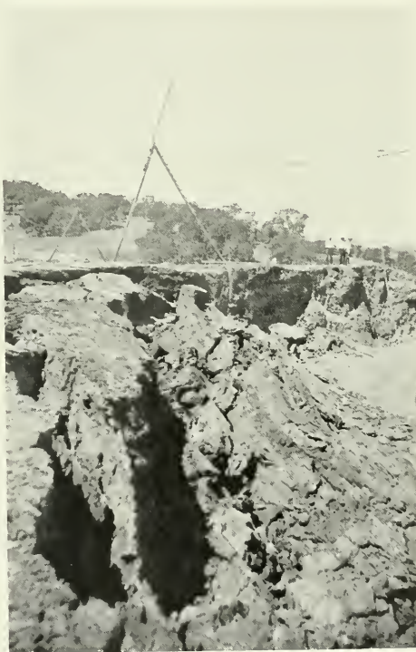
NORTH END OF BREAK NEAR CREST, LAFAYETTE DAM
