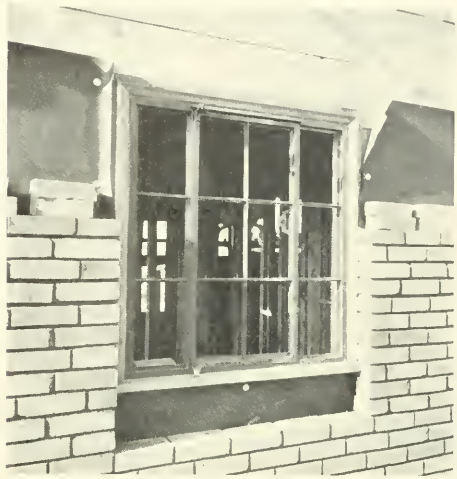
This casement is fitted with "wood surrounds" securely attached with copper-coated screws in a bed of mastic.
