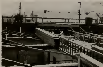
Bradford Ave School, Placentia, showing concrete struts which brace exterior walls against the corridor ceiling slab, stud bearing partitions, etc.
