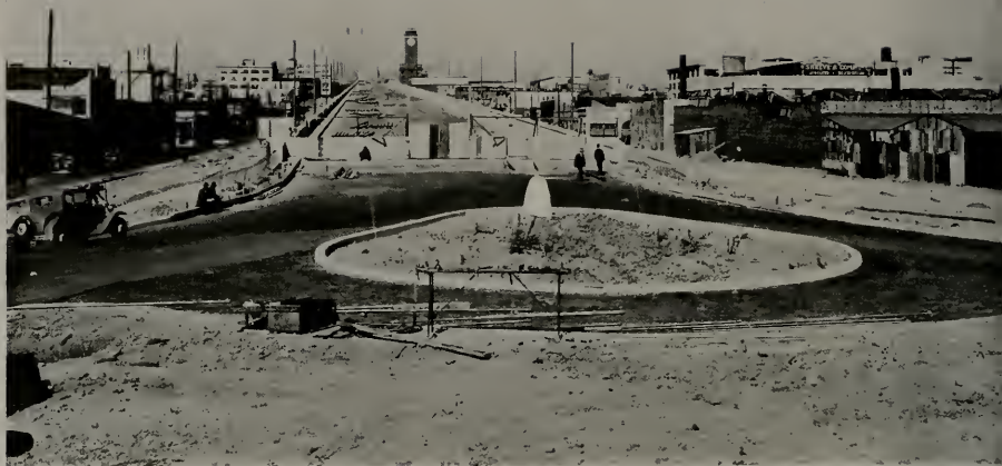
Progress work on the Fifth Street Plaza Terminal of the Main San Francisco Approach to the San Francisco-Oakland Bay Bridge. The above photograph was taken looking toward the bridge approach across the eastern point of the Plaza triangle for which an attractive landscaping design has been prepared and is now being worked out.
