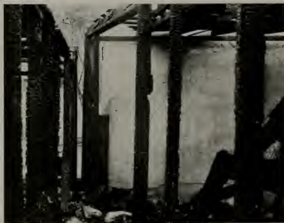
Close-up of building described above, showing badly charred studs. The white wall in the rear is the stuccoed exterior of an adjoining garage which resisted the searing flames.
