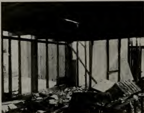
This frame building in Los Angeles was badly damaged by fire December 14. Close beside it a stuccoed garage resisted the flames, being practically immune from damage, although the heat was terrific.
