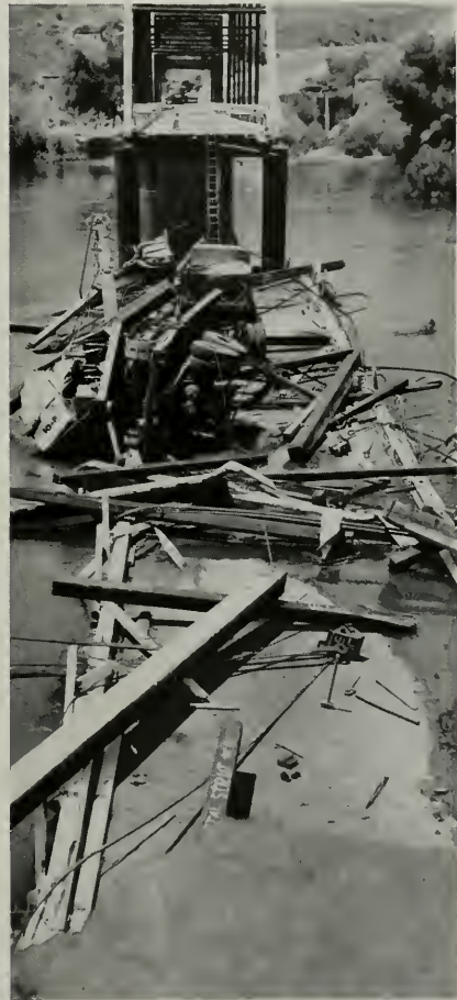
An old timber truss bridge that collapsed under a truck and trailer loaded with a power shovel, both vehicles being considerably over the posted weight limit. The truck and fallen span lie in shallow water.
