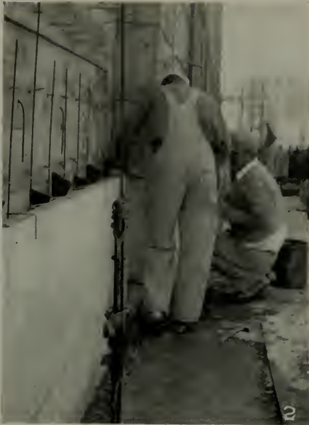
The two photographs on this page (Figures 2 and 3) show Ceramic Veneer in process of installation at the twelfth story of the Appraisers Building.
