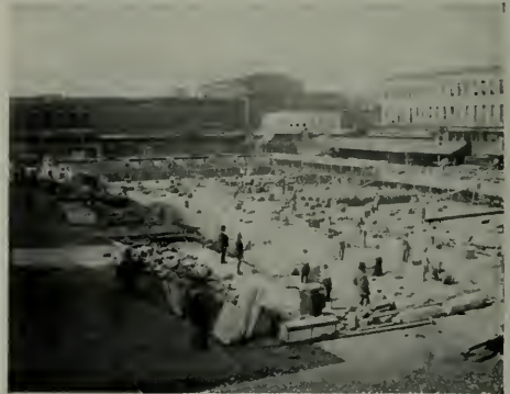
Photo shows start of construction of old Appraisers Building (1874). Note hand concrete mixers, wheelbarrows and foremen wearing stove-pipe hats to distinguish their official station.
