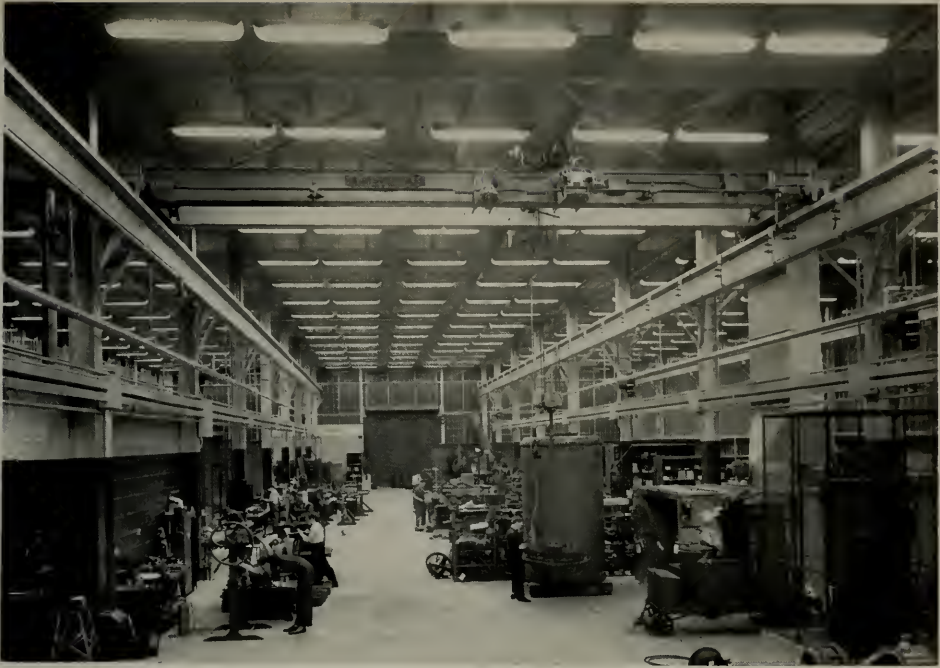
High reflection factor, white surfaces help diffuse the light and improve the efficiency of the fluorescent installation in this manufacturing and repair shop.
