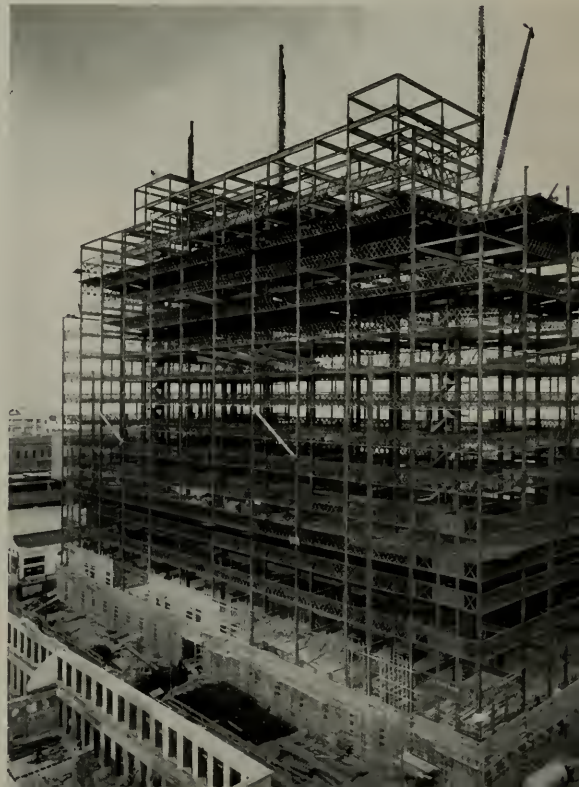
Photo shows steel frame completed. Note girder construction at each floor, a feature of the earthquake design.
