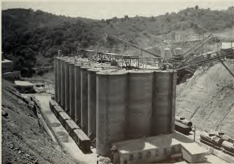
BATTERY OF CEMENT SILOS AT PERMANENTE
