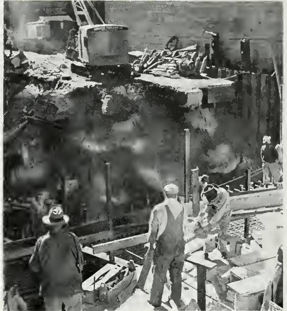
Moke-Ready-Steel mat reinforcing in foreground . . . Foundations of old five story building may be seen in center back around steel sheet piling to left and right.
