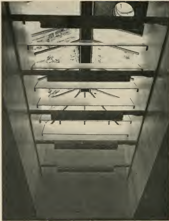
BEFORE —Unightly skylight which distorted room proportions was banked with row of baffles set to cut angle of summer sun. Fluorescent light tubes for auxiliary daytime light and indirect night lighting were placed under baffles.
