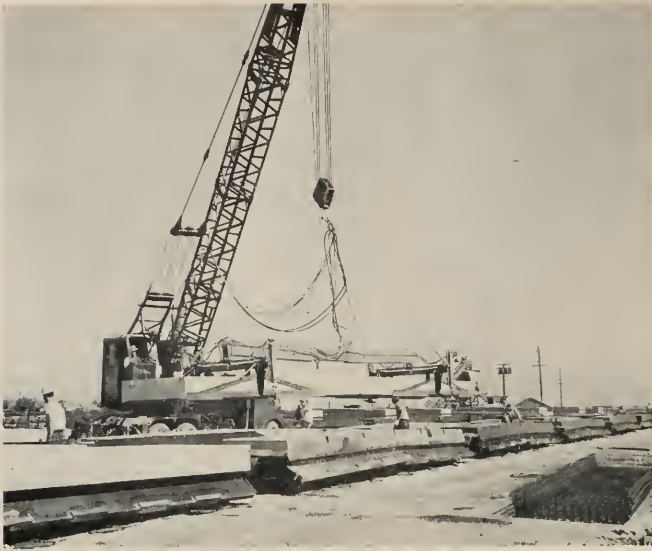
PRE-CAST , Thin shell roof panels (left) being removed from forms. Stripping process requires about three minutes.
