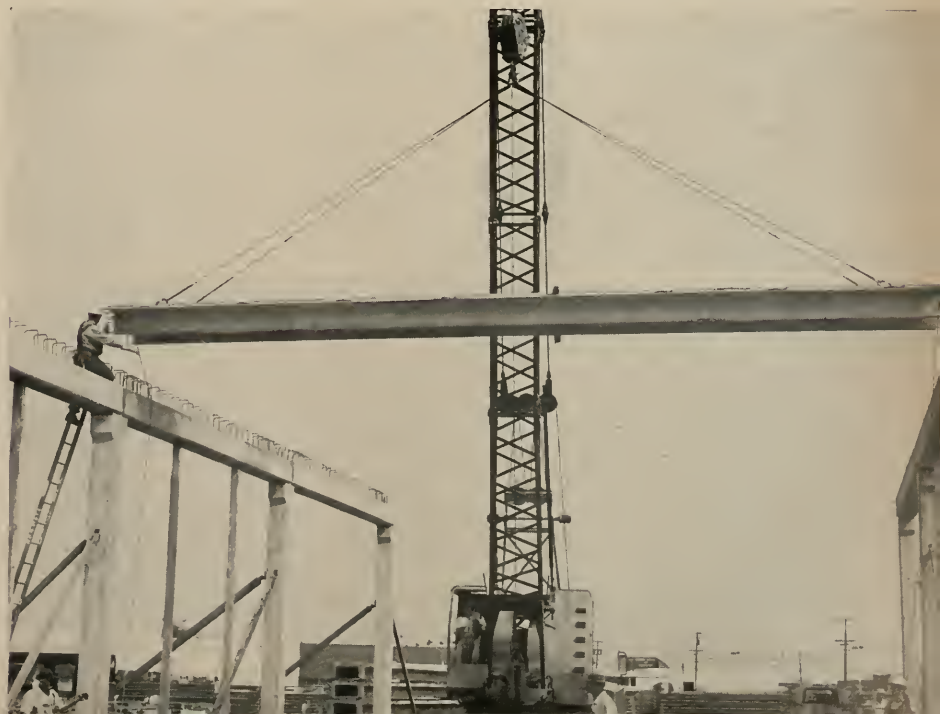
AS FIRST of 496 prestressed concrete roof panels is fitted into place. Panels pre-tensioned and cast on site in specially fabricated beds, a unique construction technique newly developed.
