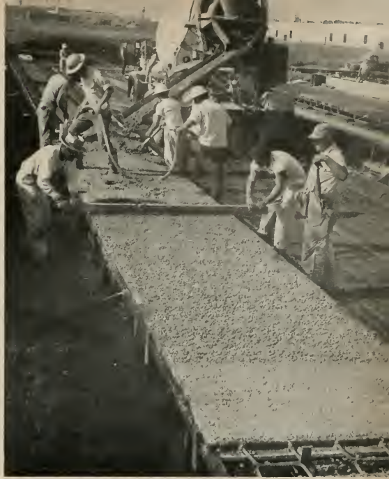
ABOVE: As the mixer truck rolls down the line, freshly poured lightweight concrete is vibrated and surface evened-off preparatory to being tamped down and smoothed by finishing crew.
