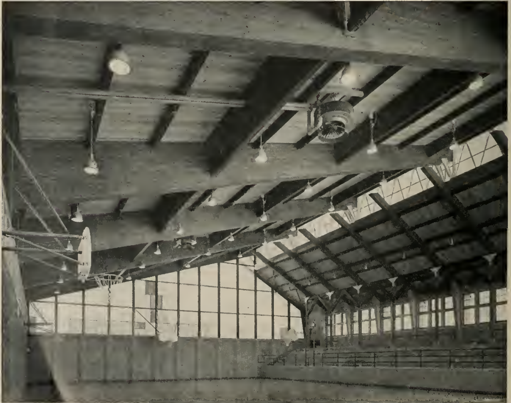
Low sloping roof section supported by cantilevered beams gives this 81 by 110 foot gymnasium illusion of smallness so children do not feel insignificant—note diagonal variable bracing.
