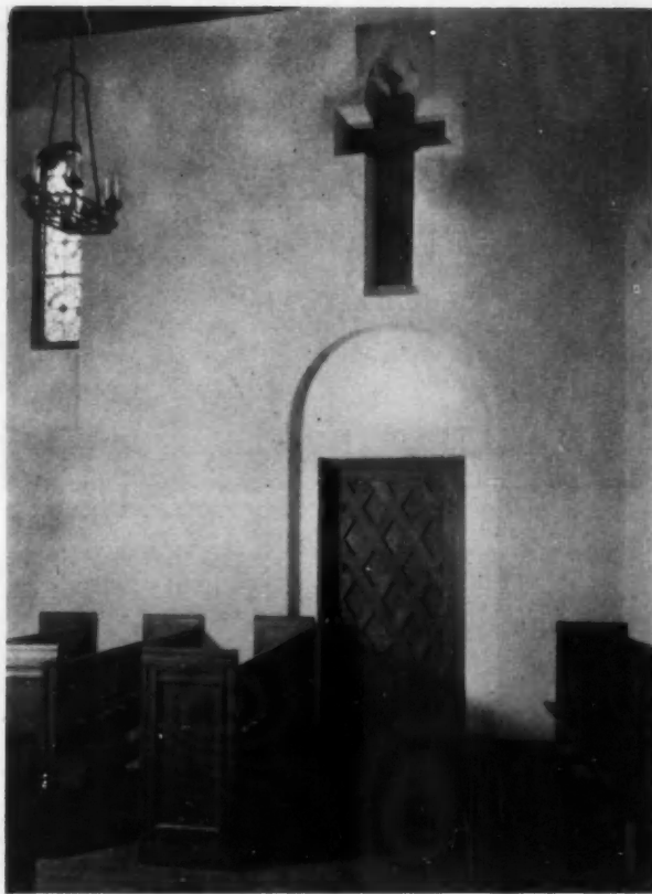
Detail of Door and Wall Penetration at the Main Entrance to the Church
